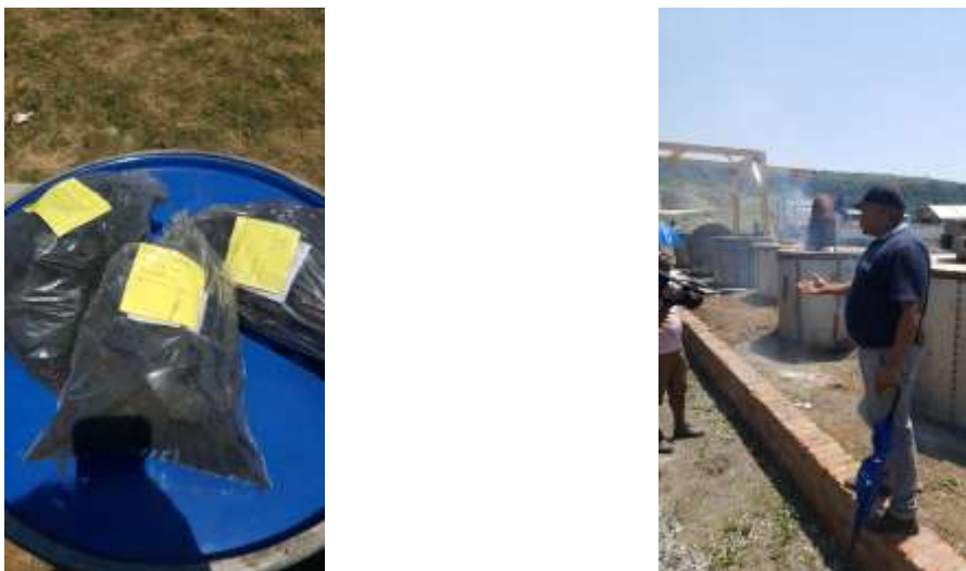
Figure 13. The East London franchising project has been exploring the decentralised disinfection and conversion of collected sludge to bio-char (left) using low-tech kilns (right). The innovation allows sludge to be treated on-site reducing logistical costs for landfill disposal.
