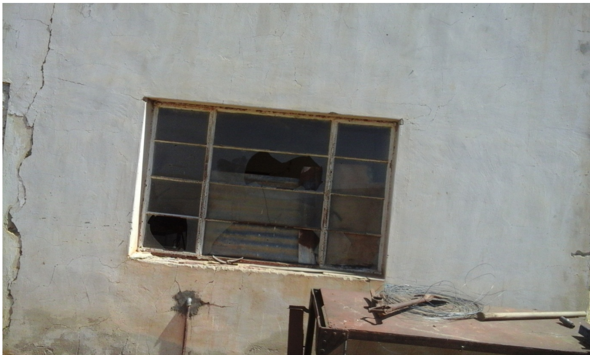
Figure 4.16: A dilapidated storage facility on a farmer's government-leased land in Barrydale, Overberg
