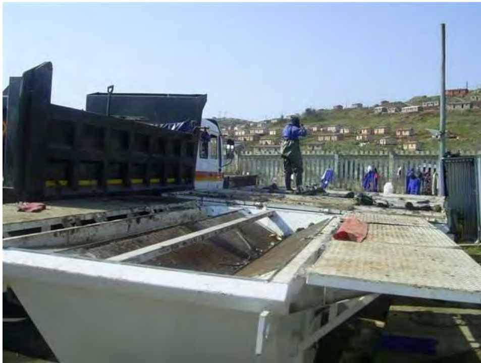
Figure 6.2 Screening trash out of sludge at WWTW (eThekweni Municipality) – it was found that the addition of pit latrine sludge at WWTWs quickly overloaded the works and this practice was discontinued
