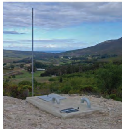
A production borehole in the Volmoed Wellfield overlooks the lower Hemel en Aarde Valley.
