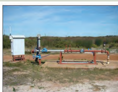
Abstraction wellhead in the Atlantis wellfield
