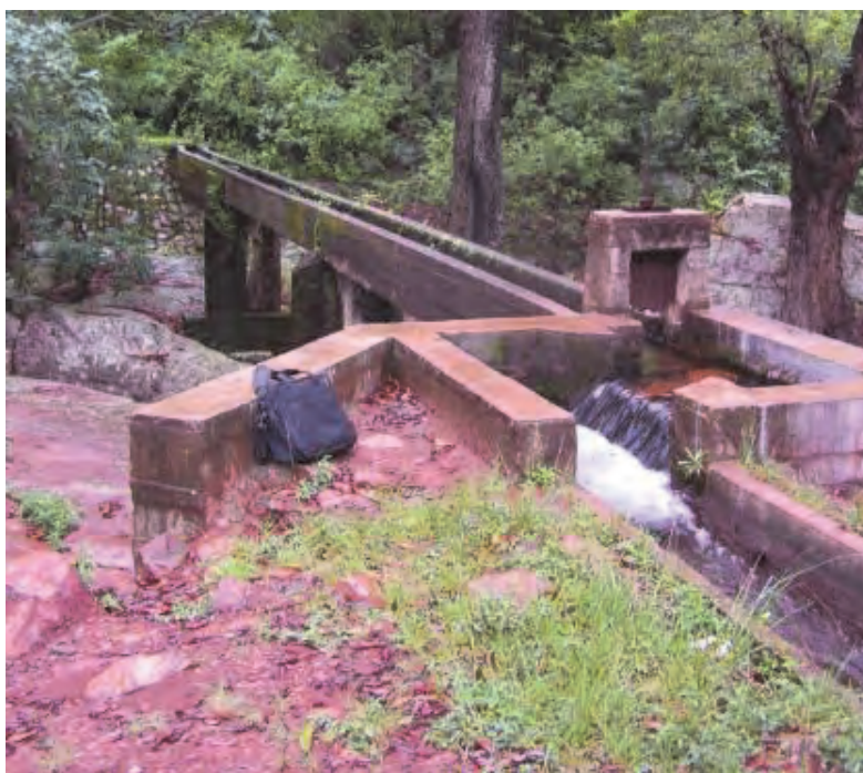
Figure 3-8 Rectangular measuring weir 200 m downstream from the Rambuda canal inlet
