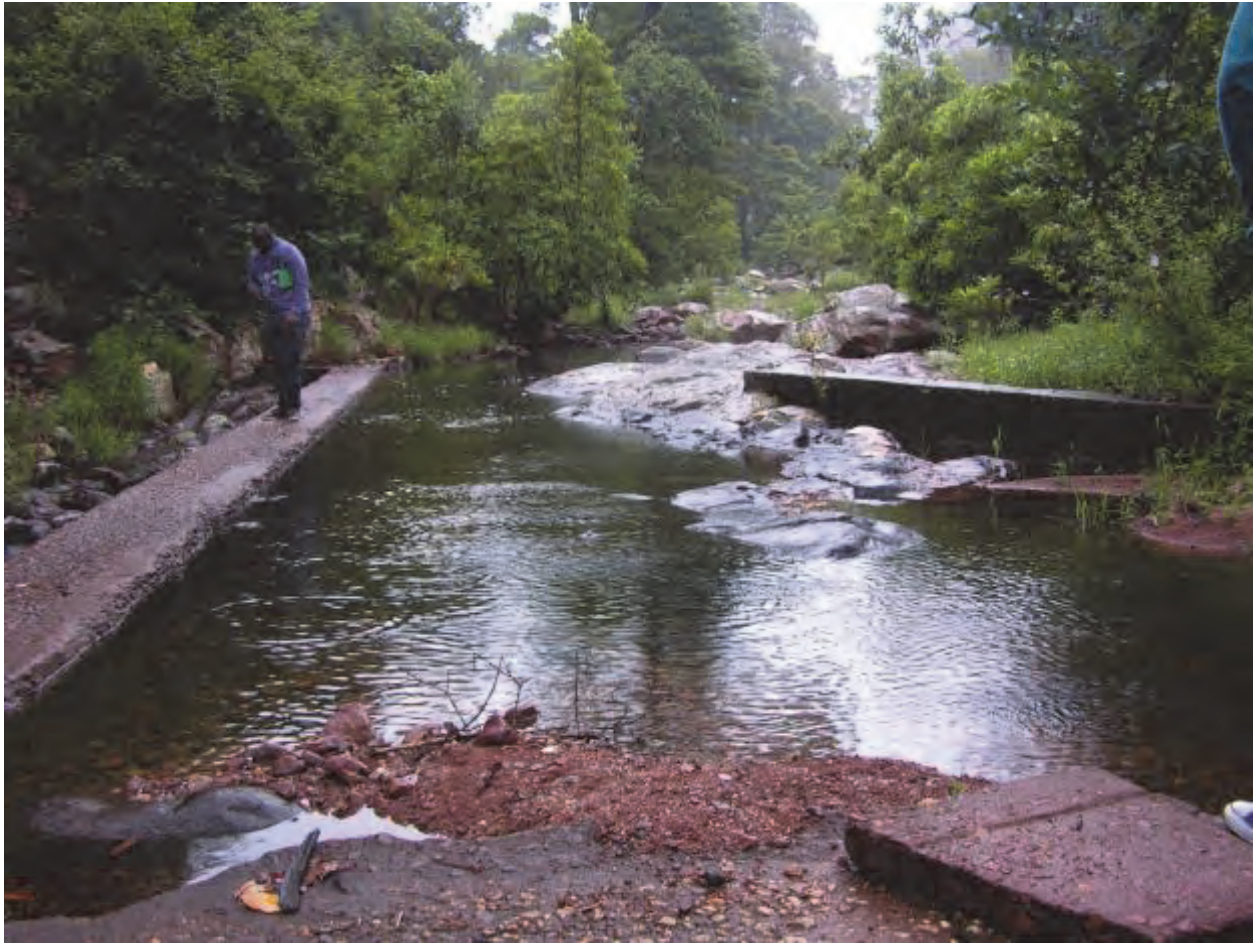
Figure 3-5 Weir in the Tshala River supplying water to the Rambuda irrigation scheme
