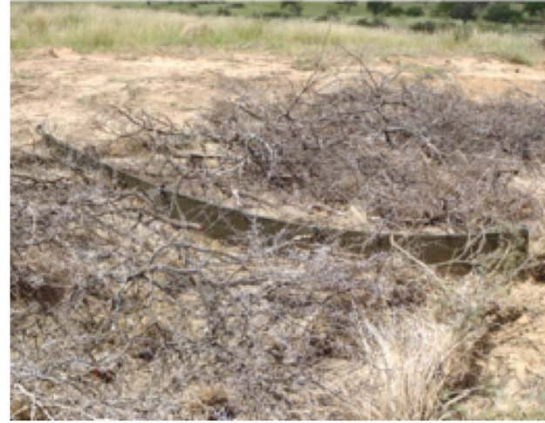
(b) GULLY SHAPING Shallow gullies less than 1 m deep can be shaped to form wider channels that can be further protected with netting or throw branches. Silt traps can be incorporated into the design.
