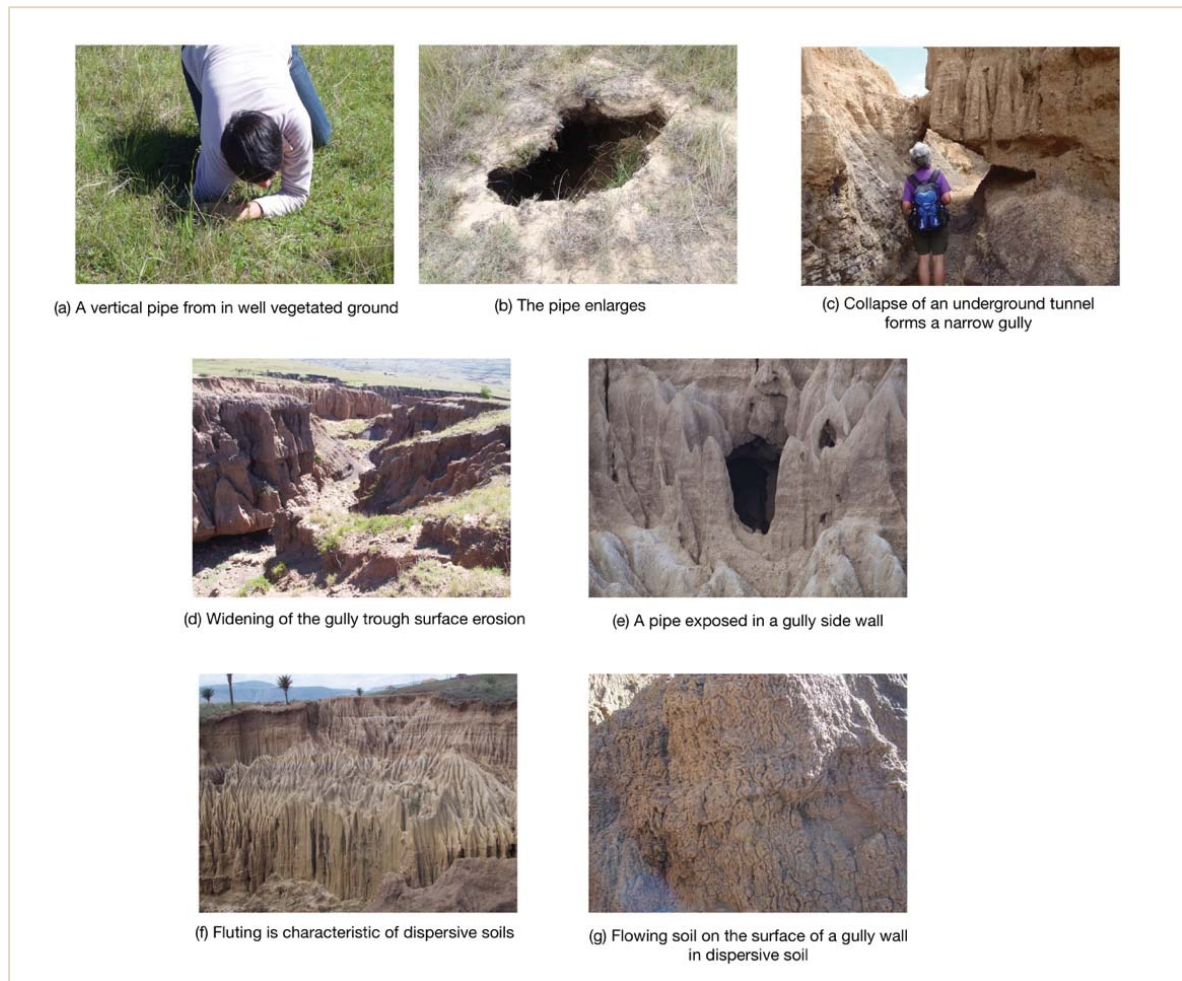
Figure 4.4: Erosion processes in dispersive soils
