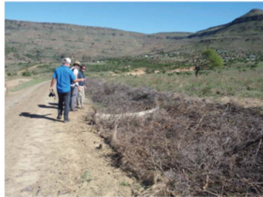
(d) TRAPPING ROAD RUNOFF Silt fences and brush packing are used here in a road-side ditch to slow down runoff and trap sediment.
