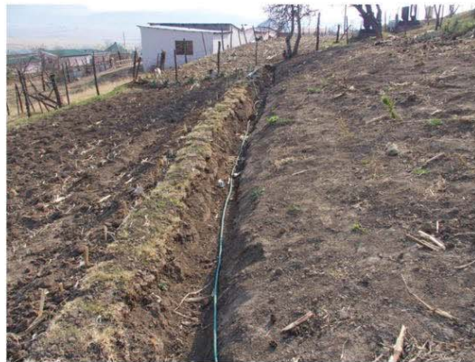
The finished swale with protective turf along the top of the downslope bund. The pipe was used to water the grass until it had become established
