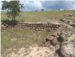
A stone pack stabilising a donga headcut
