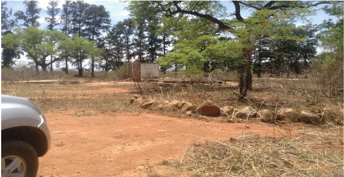
Figure 15: Vandalised office and administration block
