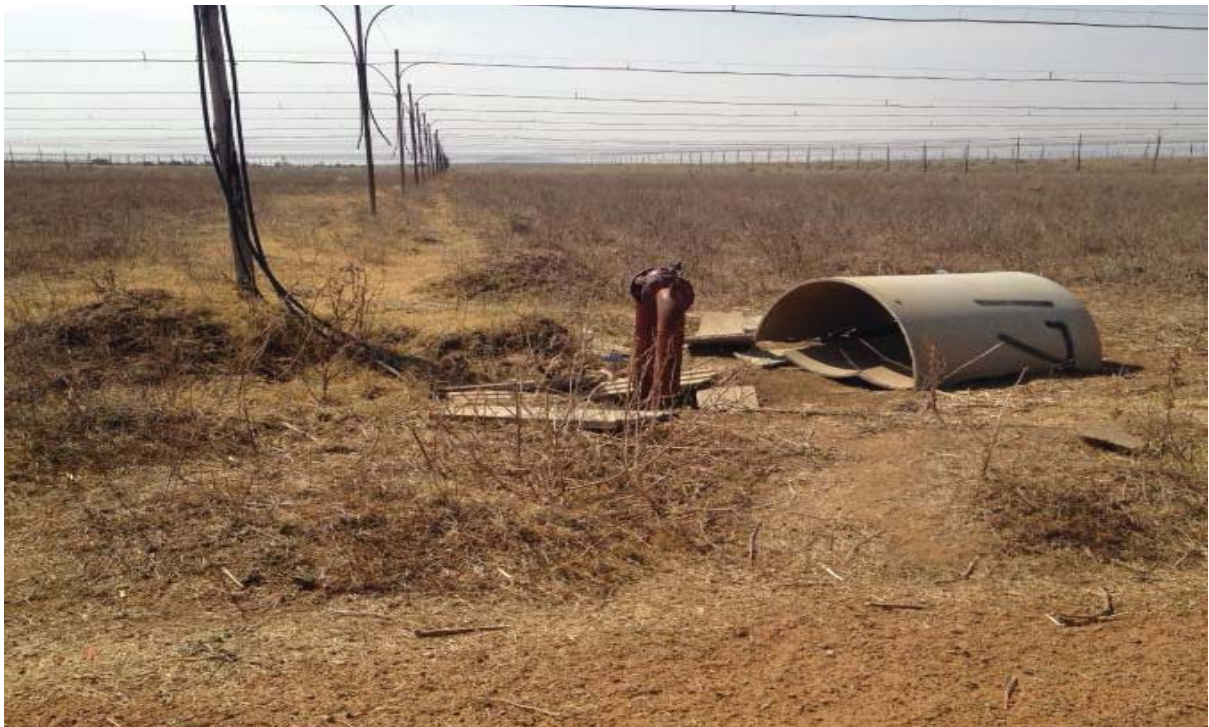
Figure 24: The manhole around this cluster valve in 2012, which now has been completely vandalized.
