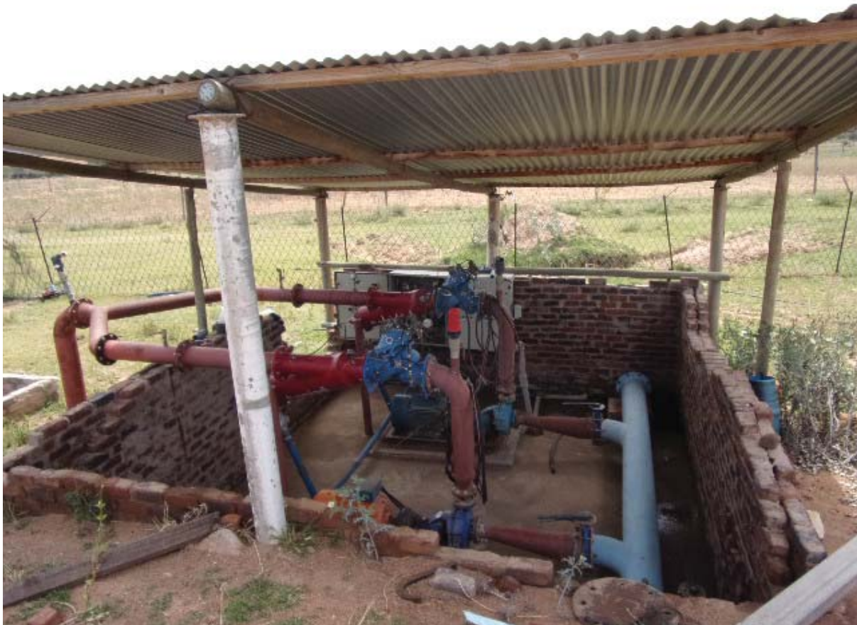
Figure 19: Poor condition of pump station at Phetwane irrigation scheme
