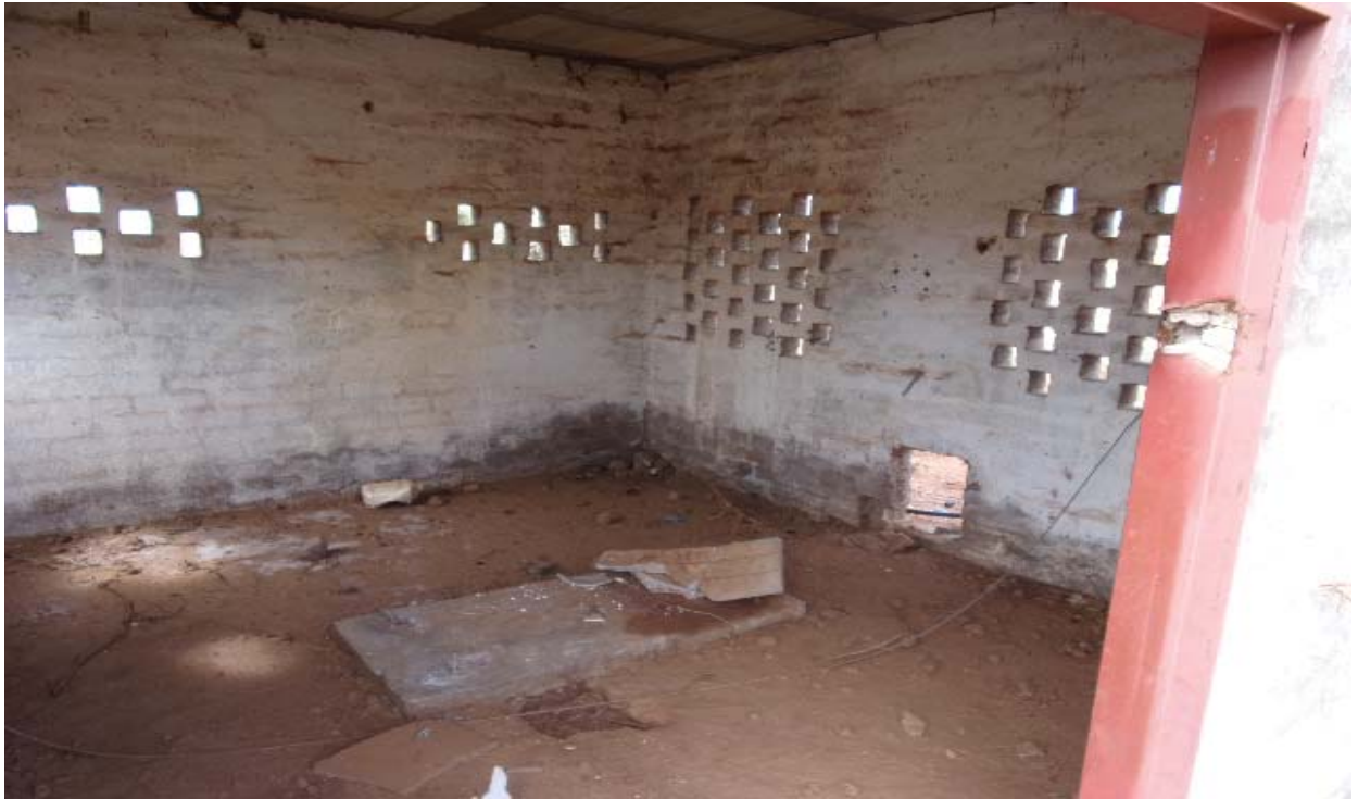
Figure 21: The original pump station which is now vandalized
