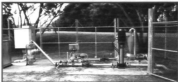
The borehole injection site adjacent to the Adelaide wetland (the borehole is on the left of the picture with the injection pipe rising diagonally to it)
