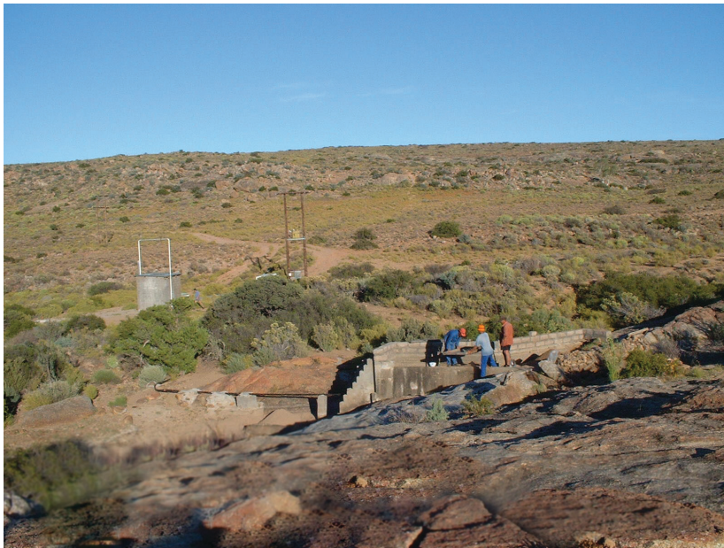
Sieving sand for rehabilitation of the sand filter. In the background is the pumphouse of the abstraction borehole.
