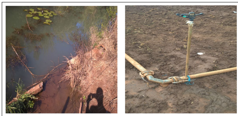
(a) Leaking canal in MRIS (b) NIS sprinkler with a makeshift component
