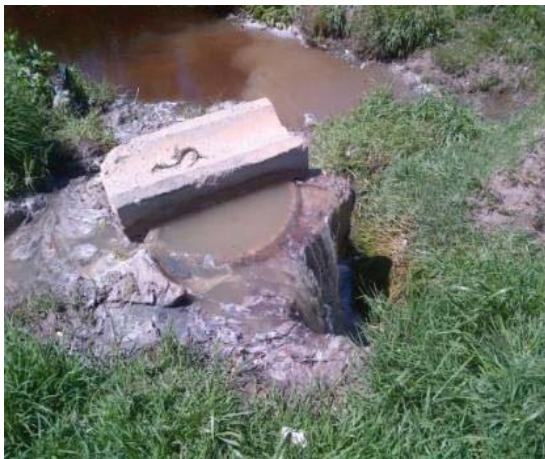
Figure 24: Raw sewage overflowing into the river
