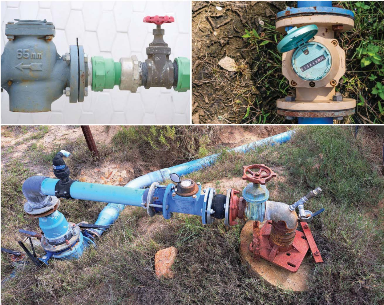
Figure 2-19 Examples of typical flow meter installations to measure groundwater abstraction from abstraction wells.
