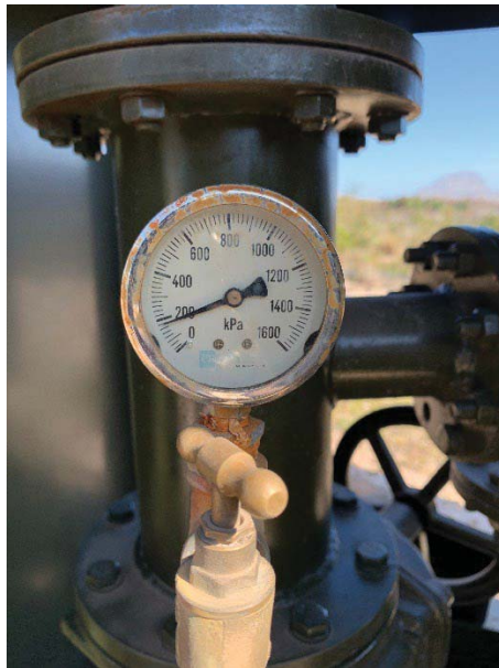
Figure 2-11 Pressure gauge fitted to a borehole that is under artesian pressure.
