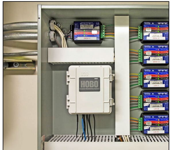
(i) Installed U30 logger
