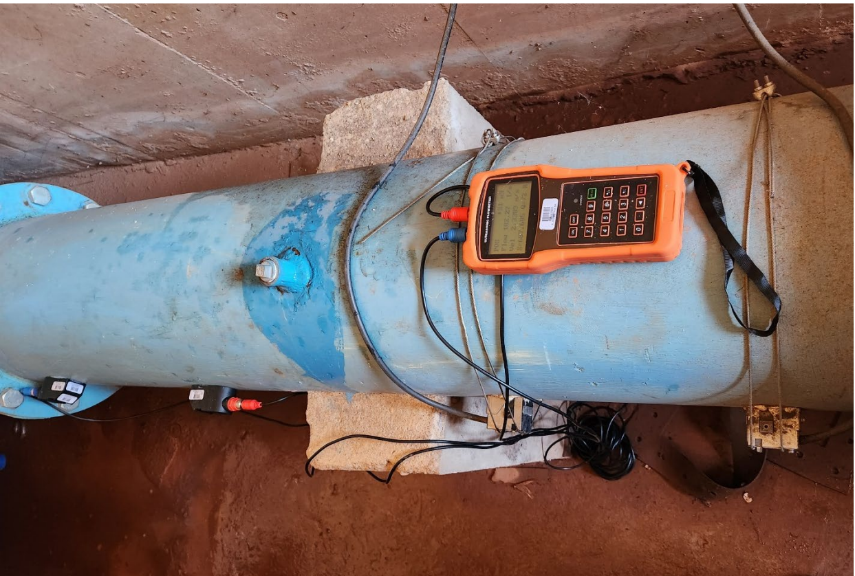
Figure 6-20: Ultrasonic flow meter installed in Chamber C on inlet pipeline for additional verification of flow meter C-FM (407)
