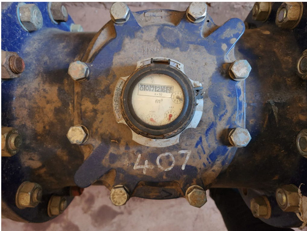
• Figure 6-25: Inlet flow meter - C-FM (407)
