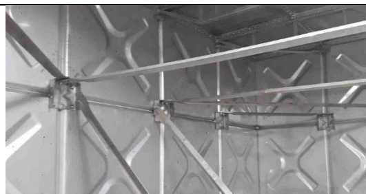
Internal supports, steel reservoir tank
