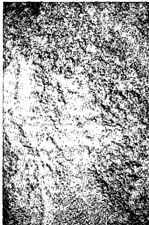
Figure 4f Fresh scum breaking through hard layer of sludge on surface of sludge return channel
