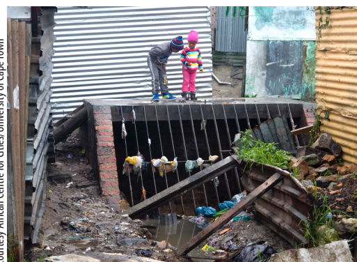
This drain is part of a stormwater management system, put there to siphon off the water that fetches up in a 'detention pond', a manmade wetland built to hold water temporarily after heavy downpours. But, since the pond stands dry during summer, desperate people set up their homes on what seemed like suitable open ground, often not knowing what the winter months would bring.
