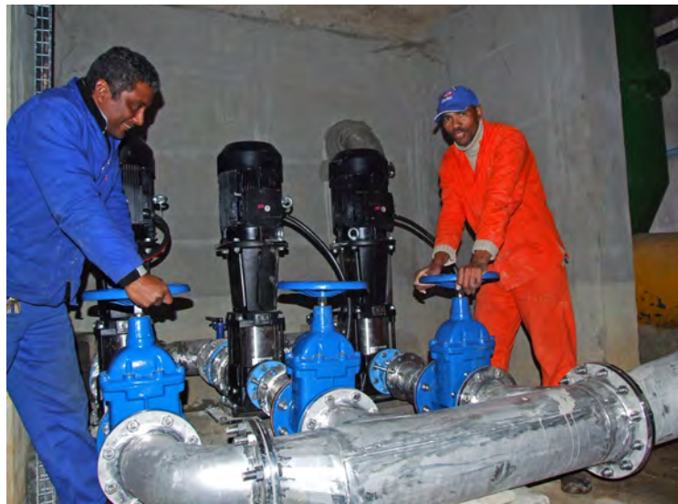
The Lelifontein booster pump at Wellington was upgraded as part of Drakenstein’s water demand management efforts.
