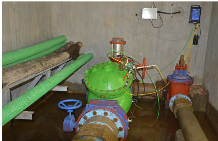
A pressure management installation in Paarl. Pressure management has had the largest impact on reducing Drakenstein's water demand.
