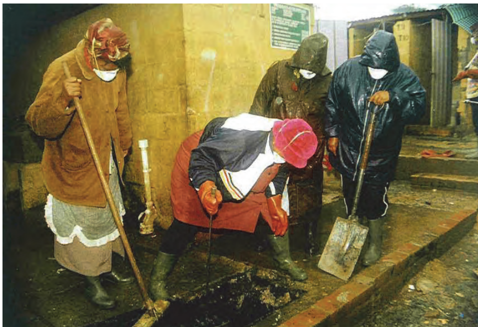
Part A: Community members being trained in the unblocking and repair of drains around the communal toilet blocks. All these trainees received their basic certificates in plumbing from the training team of the Department of Labour.
