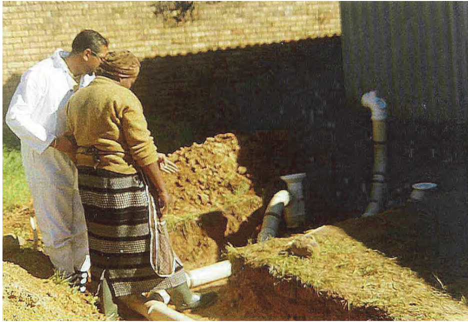
Part A: One of the members of the Kayamandi community who received training in plumbing during the project. The plumbers who were trained were meant to help with the upkeep of the communal toilet facilities.
