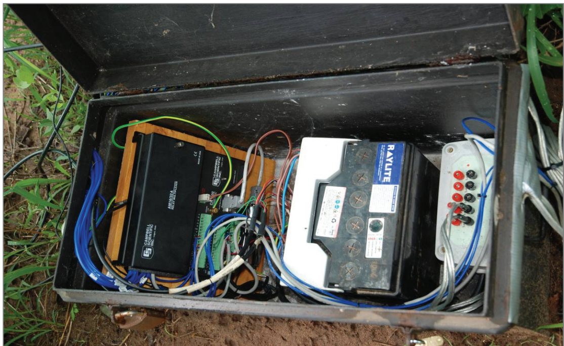
Plate 7.10 HPV Data logger, multiplexer, relay control module and battery
