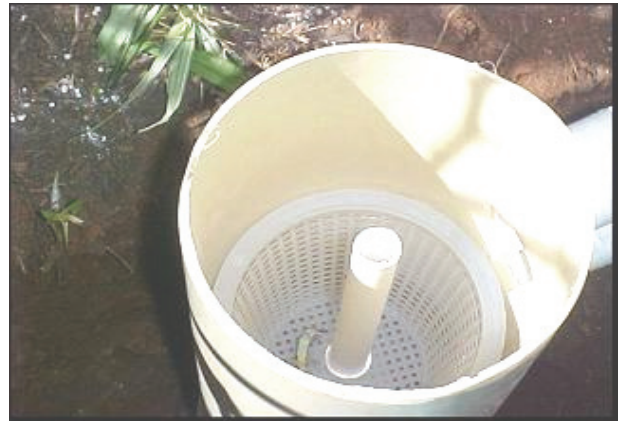
Figure 9. Grey water filter and sump
