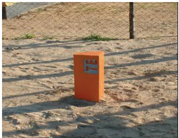
Figure A11. Orange colour coded pipe marker
