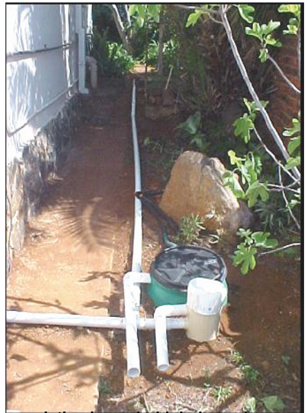
Figure 15. An example where plumbing for an existing household drainage is retrofitted into the grey water reuse system
