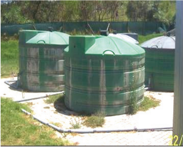
Figure 19. The primary treatment facility
