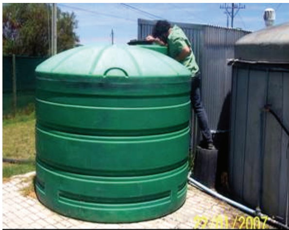
Figure 20. The treated effluent storage tank
