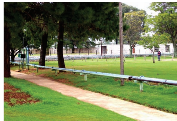
Figure 35. A dual treated effluent (green pipes) and potable (blue pipes) water reticulation within the Training Centre.
