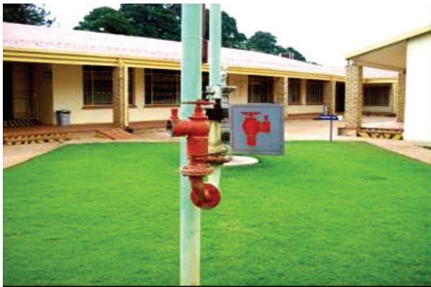
Figure 34. Green colour pipes conveying treated effluent for irrigation at the Training Centre.
