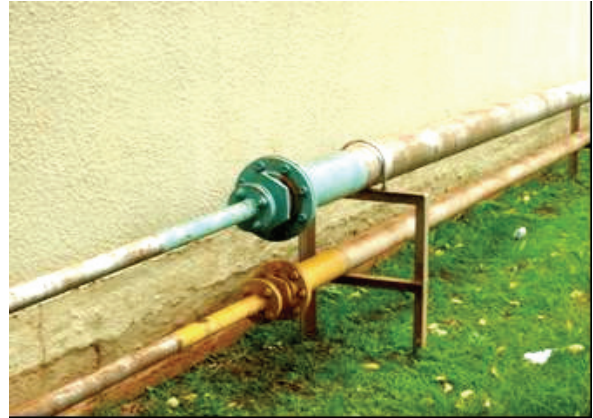
Figure 33. Pipes supplying communal toilets**
