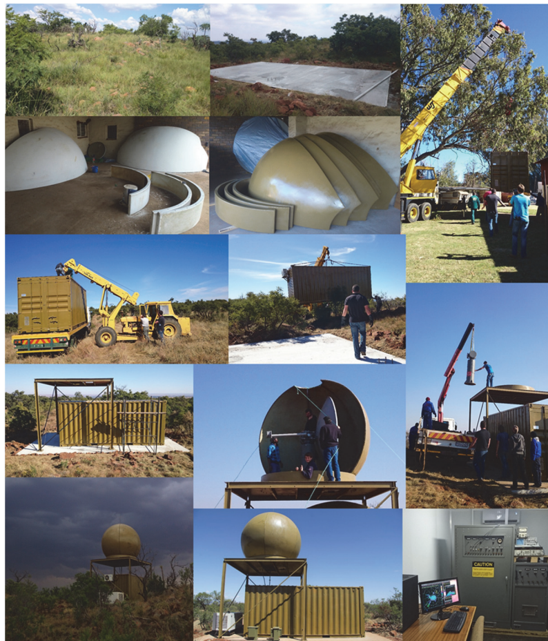
Figure 2.30: A mosaic of the NWU Lekwena radar installation.
