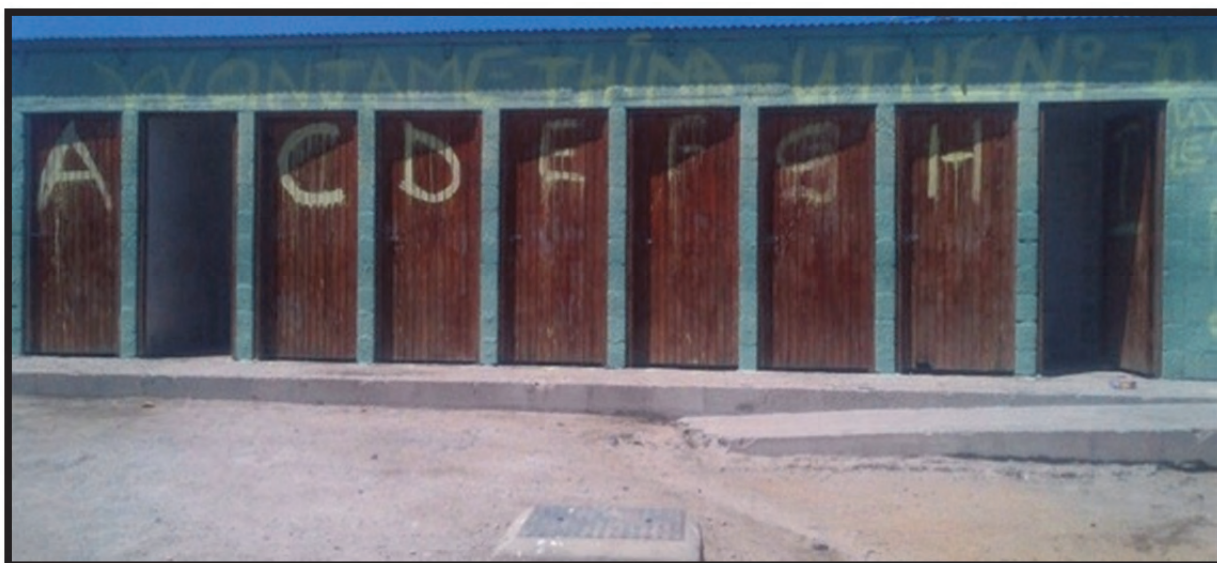
Figure 4-8: A brick and mortar toilet block in Zwelihle's Transit Camp is raised to prevent the toilet cubicles from flooding (Vice, January 2013).
