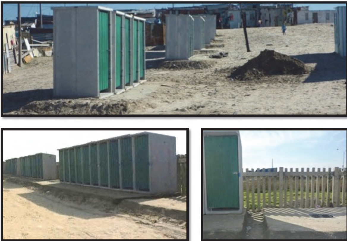
Figure 3-15: The new toilets in BV Section were built on raised concrete platforms in open spaces between residents' homes (top), and alongside a dirt and gravel road (bottom-left). For the latter, drains were also installed in the concrete platforms and channels were created between each platform to allow for stormwater drainage either into the reticulation network, or the N2 road reserve behind the palisade fencing (bottom-right; Taing, June 2013).
