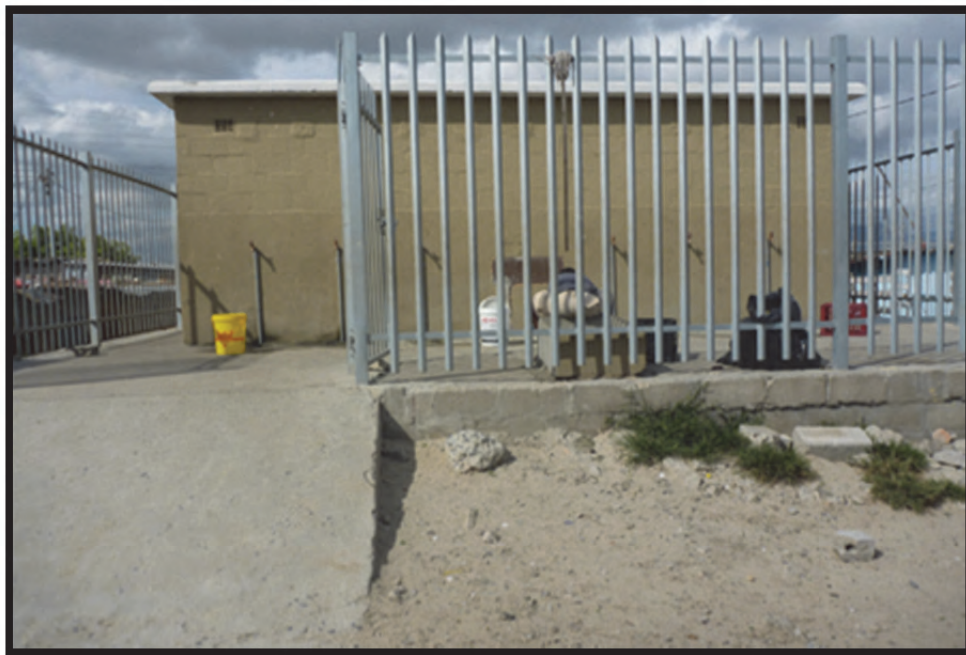
Figure 3-13: The BM ablution block (Taing, March 2013). Residents use the seven standpipes alongside the front of the building to wash their hands and to fill buckets. Residents often wash clothes in the open area next to the standpipes.
