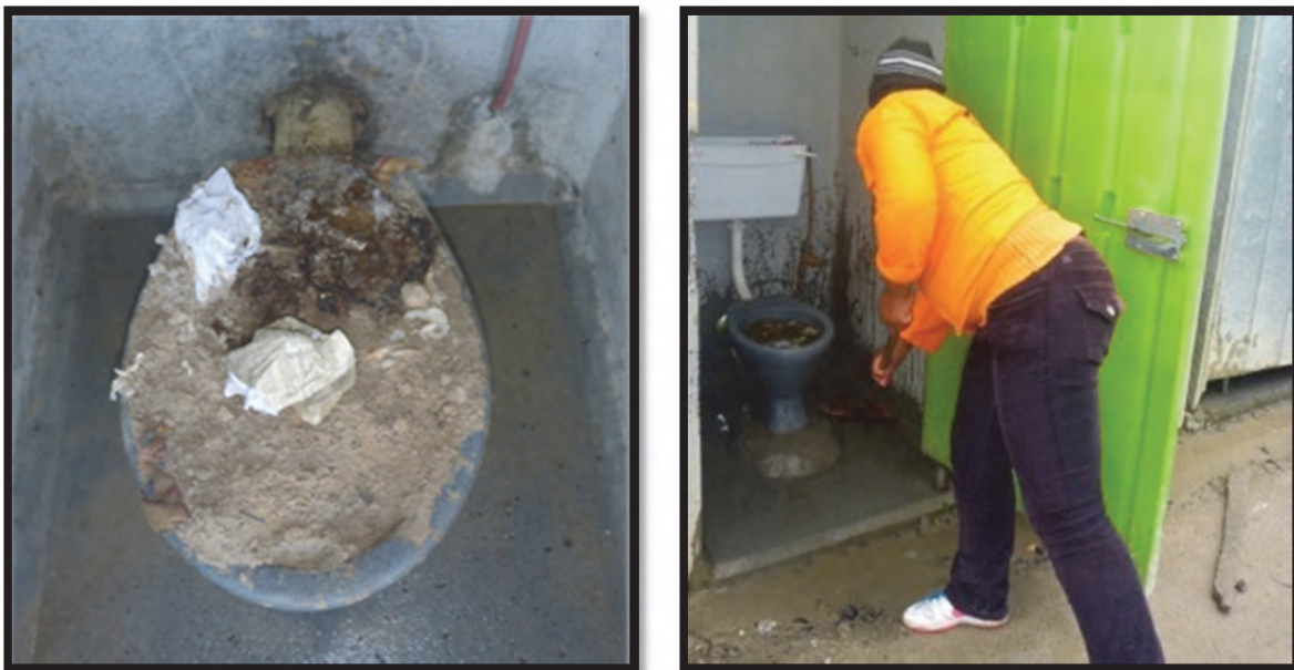
Figure 3-27: Pictured on the left is a dysfunctional toilet that janitors said they filled with sand to cover the smell of decomposing waste and so that residents would not use the units (Taing, July 2013). Evidence of human waste in broken toilets indicated that people continued to use these facilities. The bottom of this unit is wet because a janitor had just swept it. The photograph on the right shows a janitor sweeping the floor of a blocked toilet.
