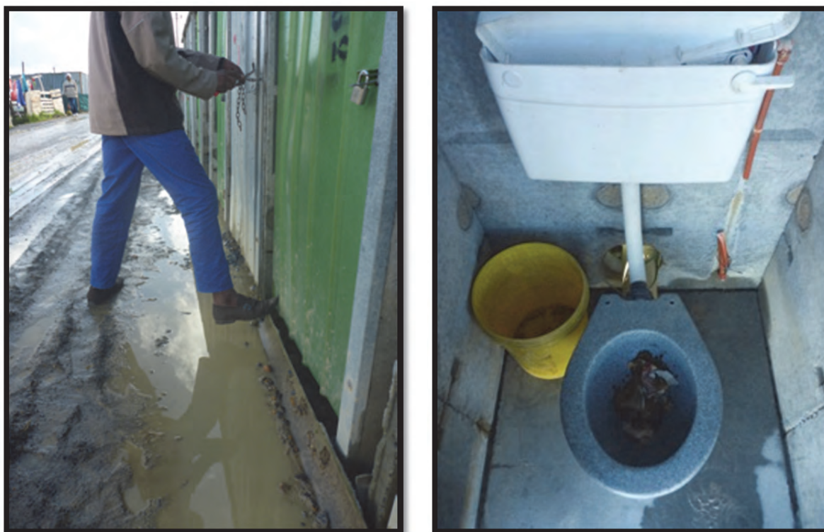
Figure 3-12: A resident carefully avoids the stormwater that pooled in front of the toilet he uses in BM Section (left). It was observed that some people continued using toilets in which the water supply was cut by utilising buckets to flush the bowl (right) (Taing, June and May 2013).
