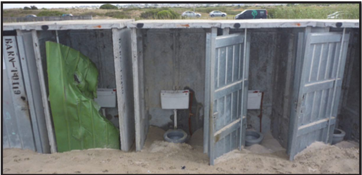
Figure 4-7: Residents in Zwelihle, BM Section and Masiphumelele said they often struggled with sand, rain and wind when using clustered flush toilets away from their home. Though an extreme example, these disused toilets in the fire-affected area of BM Section show how facilities such as these are often fully exposed to the elements and offer users/janitors little shelter during inclement conditions (Taing, January 2013).
