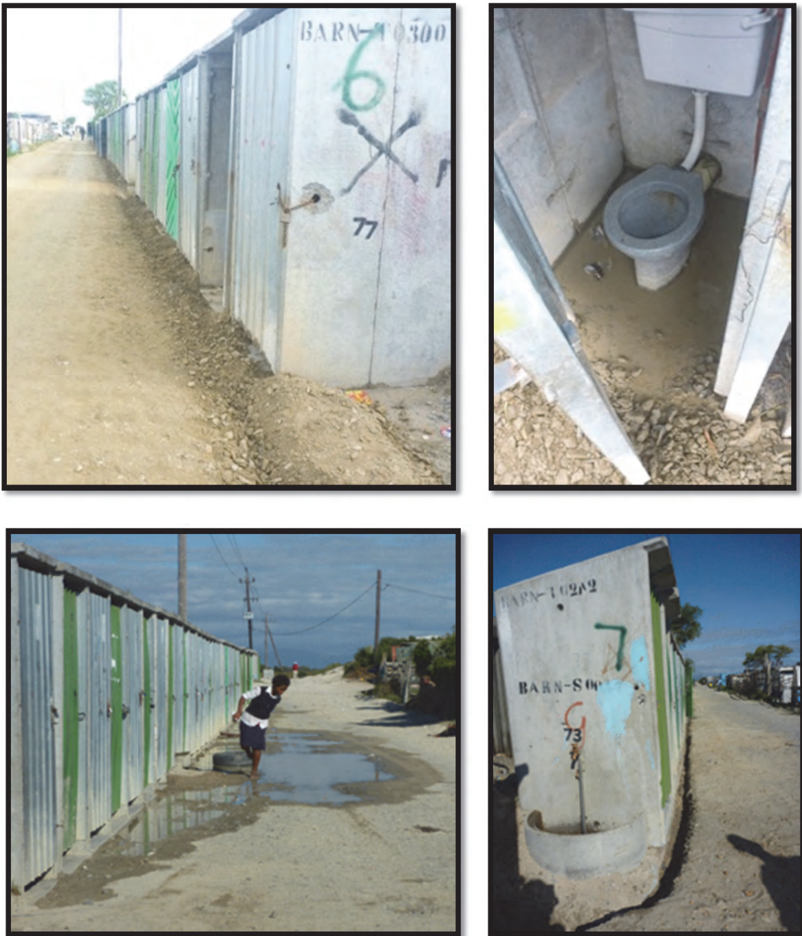
Figure 4-14: Clockwise from left to right): WSISU Officials said that CoCT's Roads and Stormwater raise the gravel road by the N2 toilets in BM Section annually, which has meant that over the years these toilets are at a lower level than the road, and (a) get flooded regularly due to stormwater runoff from the road, or (b) when the water from leaky cisterns pool (Taing, May 2013). Janitors reduced the amount of standing water in the units by (c) creating ditches that drained water, so that (d) users did not have to jump over pooled water or use waterlogged toilets (Taing, February 2013).
