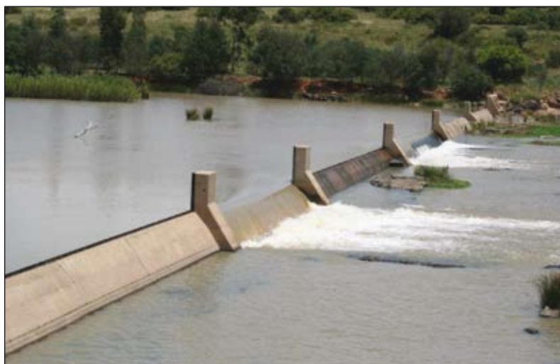
Figure 6 Example of a compound sharp-crested weir in the Vaal River downstream of Vaal Dam
