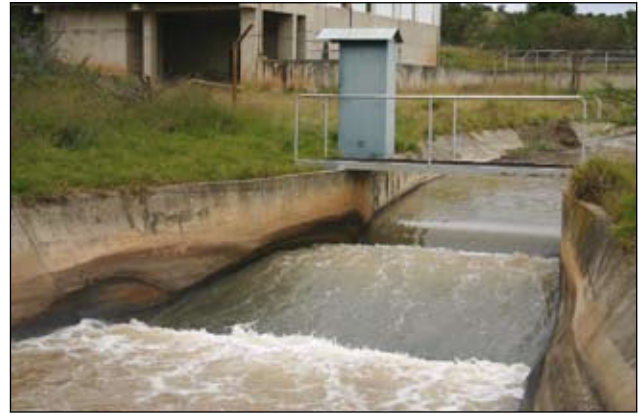
Figure 14 Example of a Parshall flume installed in an irrigation canal
