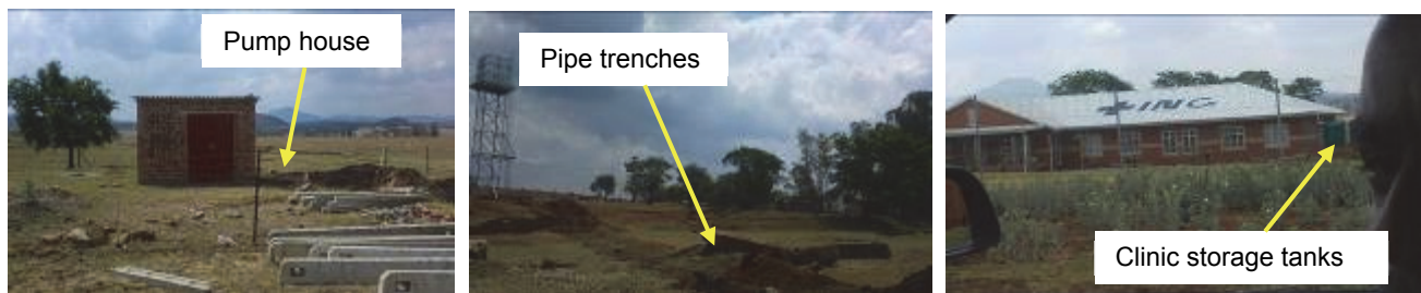
Figure 3.28: Ingogo Section 2 community water system photos
