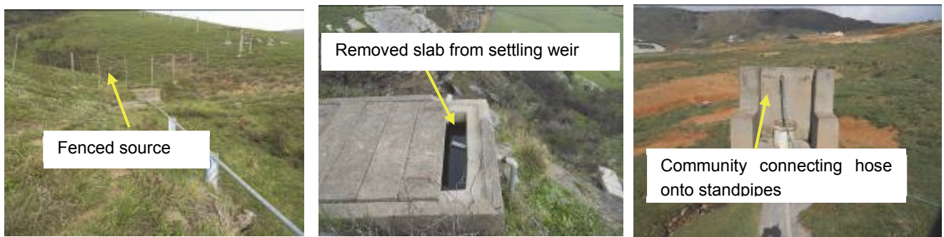
Figure 3.6: Nyibibeni community water system photos
