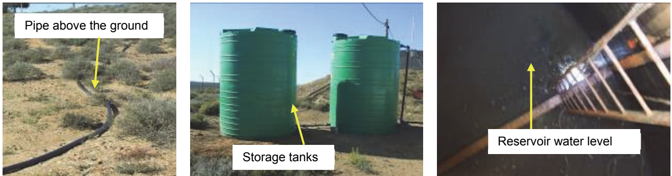
Figure 3.22: Loeriesfontein community water system photos
