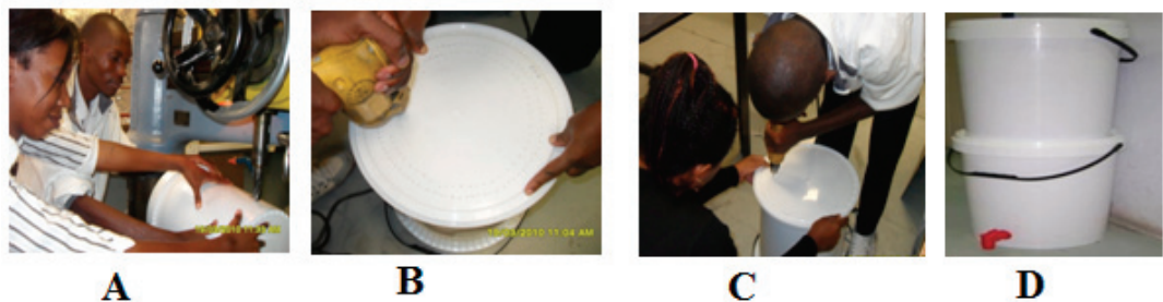
Figure 4 Steps for preparing buckets for the construction of a bucket filter: A – Drilling of hole to fit spigot; B and C – Drilling of holes on the lid of the bottom bucket through the base of the top bucket; D – A complete bucket filter.
