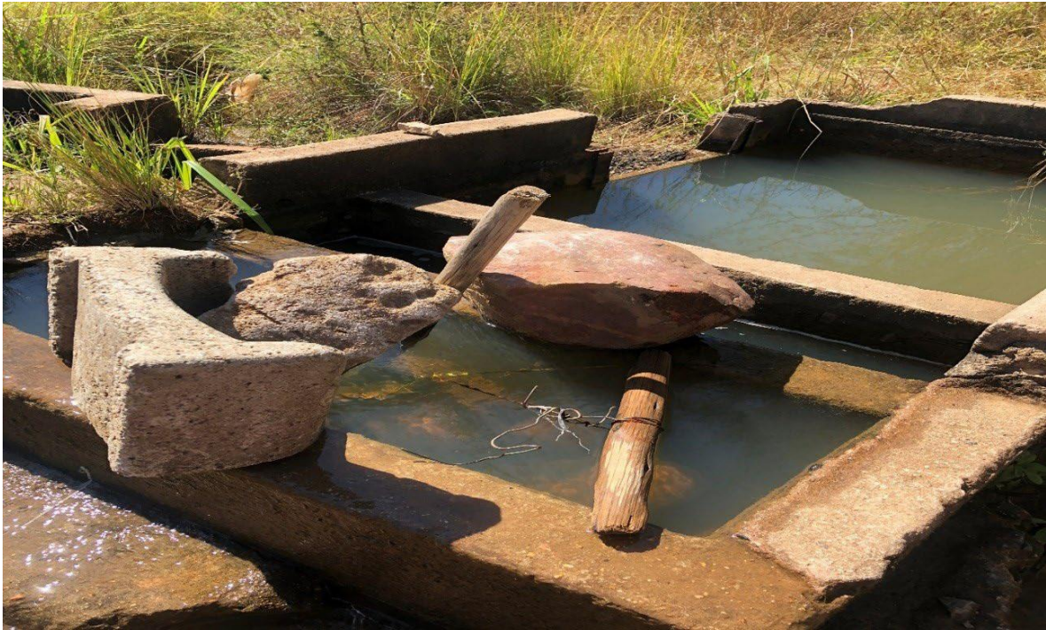
Figure 7. Major challenges with canals at New Forest irrigation scheme Source: Fieldwork 2021
