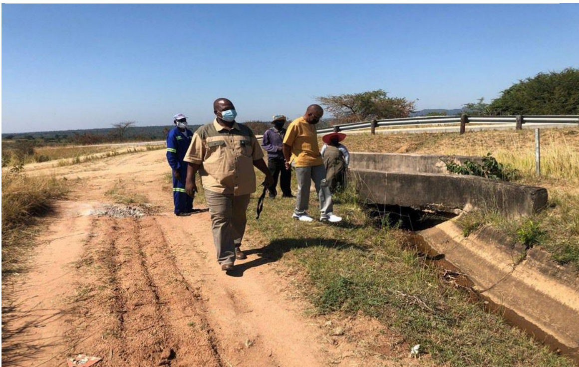
Figure 8. Major challenges with unmaintained/damaged canals at New Forest irrigation scheme Source: Fieldwork 2021
