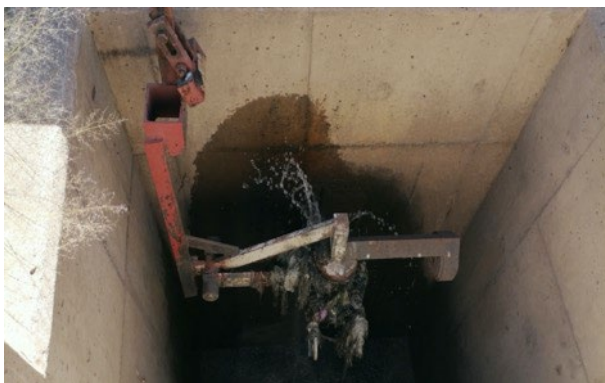
Figure 15: Scum removal valves overburdened with debris
