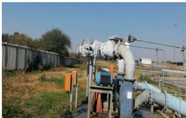
Figure 78: Leak at the sludge pump has created a serious spillage
