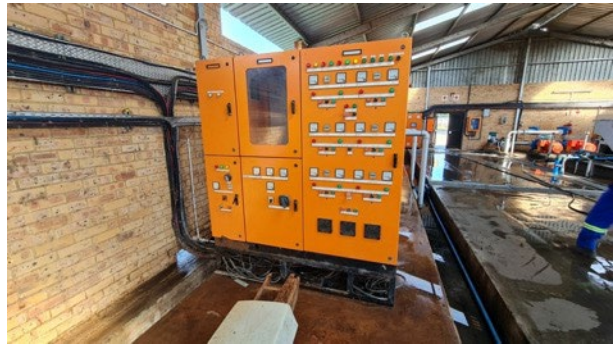
Figure 55: Old MCC for sludge pumps, polymer station found not working
