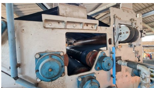
Figure 48: Dewatering belt press No. 1 working, but one belt is severely torn
