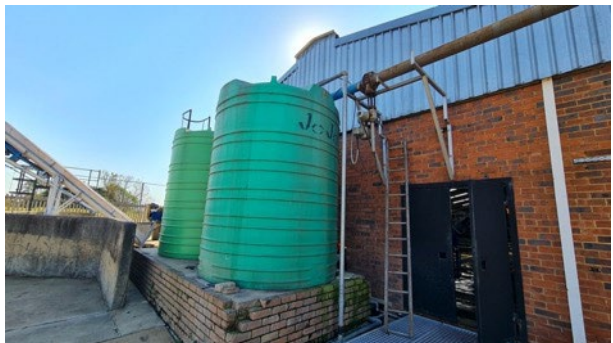
Figure 53: Wash water storage tanks seen to be functioning and in a fair condition
