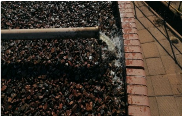
Figure 69: No End-Caps on some filter arms
