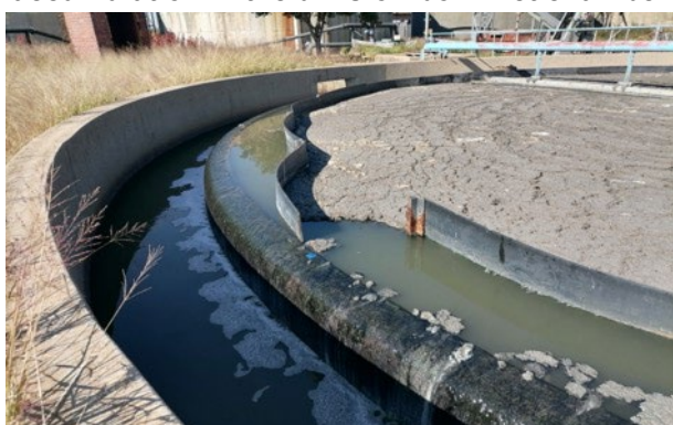
Figure 25: Broken scum baffle resulting in scum overflowing to the biofilters
