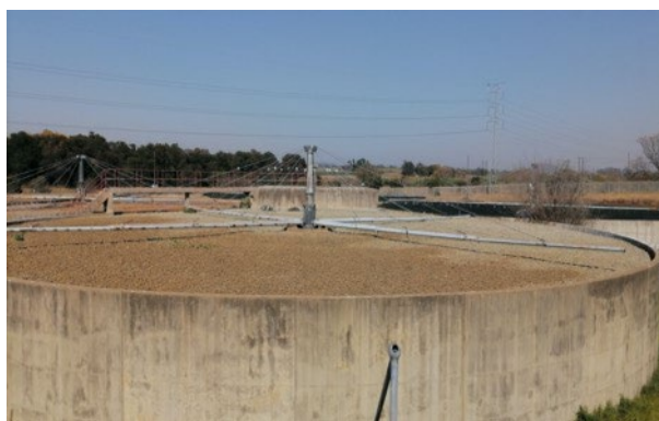
Figure 28: Filter out of commission for a long time due to faulty centre column
