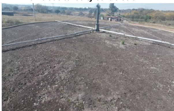
Figure 30: A layer of sludge observed in one of the filters out of commission
