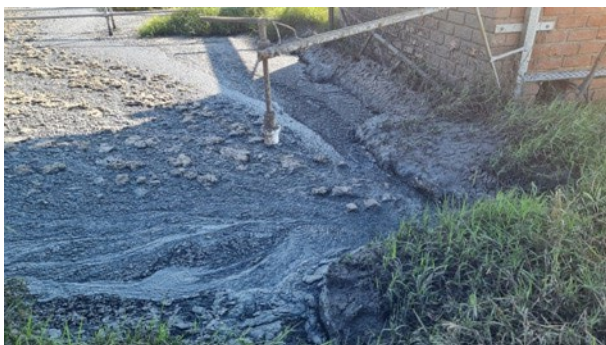
Figure 44: Northern sludge handling plant inlet sump overflows to nearby fields
