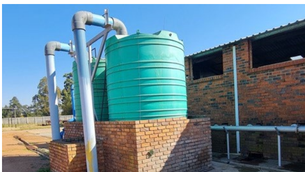
Figure 46: Buffer storage tanks before belt presses
