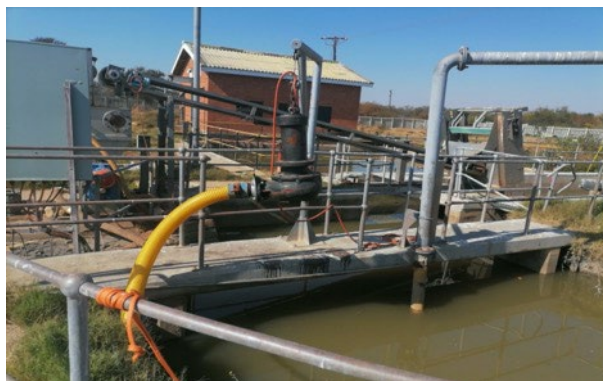
Figure 66: The only available grit pump removed for repairs
