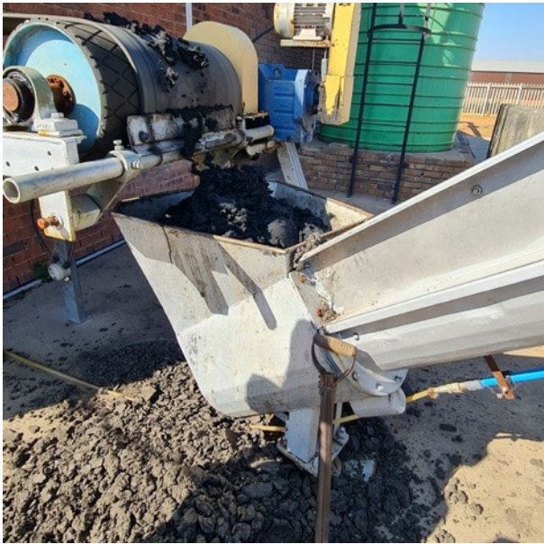
Figure 50: Dewatered sludge overflow at screw conveyor
