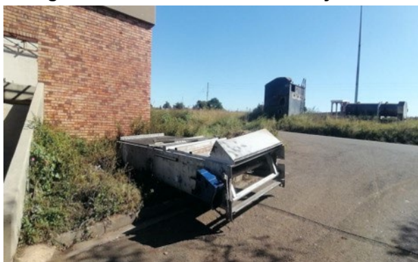
Figure 5: One of the mechanical screens left unattended
