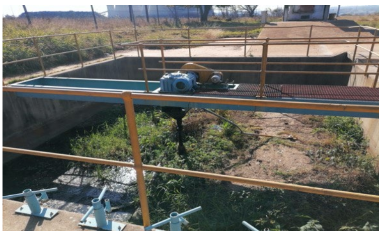
Figure 22: One grit chamber out of commission for a long time
