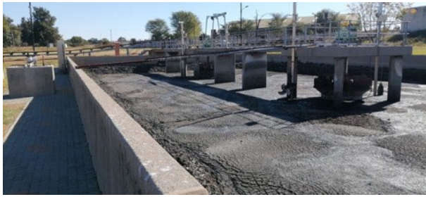
Figure 58: Sludge handling sump one with mixers and aerators that do not work. A top layer of scum was seen
