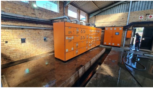
Figure 54: Sludge dewatering plant MCC and control panel in a working condition
