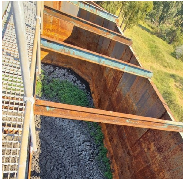
Figure 51: Elevated dry sludge hopper at an extremely low level
