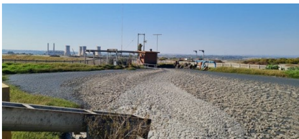
Figure 42: Accumulation of scum at the sludge handling sump
