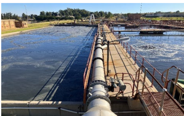
Figure 11: Leaking pipework in the diffusers
