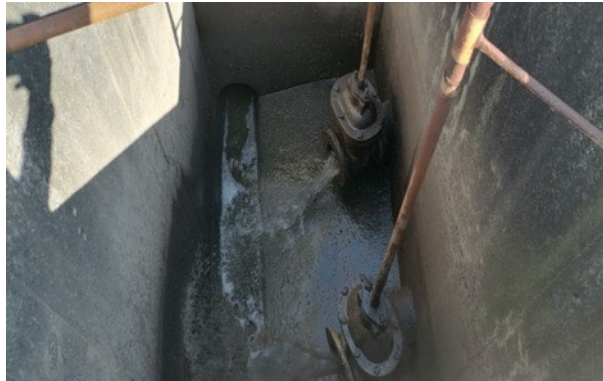
Figure 33: Scum and sludge removal valves always left partially open for no apparent reason
