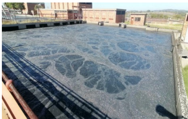
Figure 10: Foaming in the aeration basin
