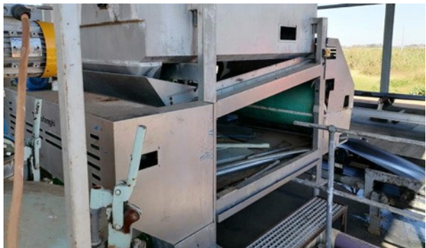
Figure 61: Sludge dewatering belt press used for spares
