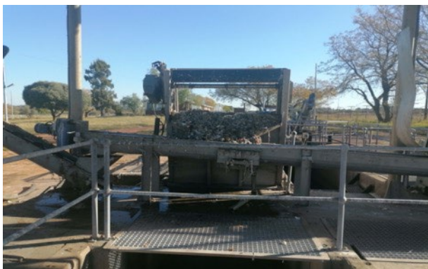
Figure 20: Condition of inlet screens
