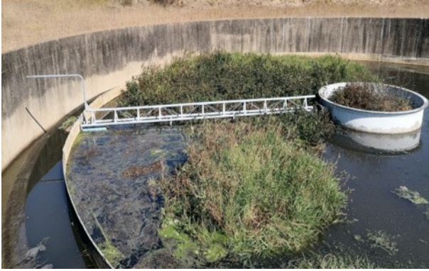
Figure 31: Poor conditions apparent in most humus tanks
