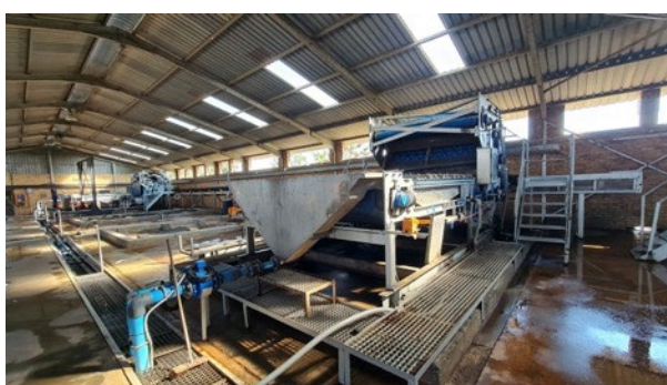
Figure 49: Dewatering belt press No. 4 out of commission and two other belt presses removed
