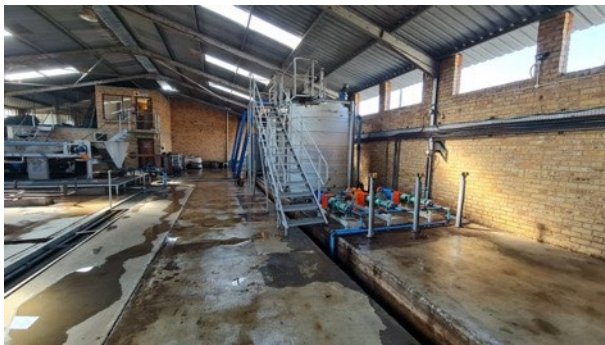
Figure 56: Polymer dosing station and pumps are functioning and in a fair condition
