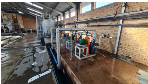
Figure 47: Pump station for two out of four belt presses installed and correctly functioning
