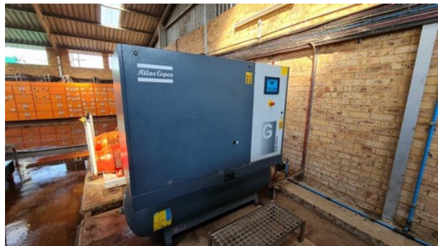
Figure 57: Compressor for sludge dewatering belt press works and is in a fair condition
