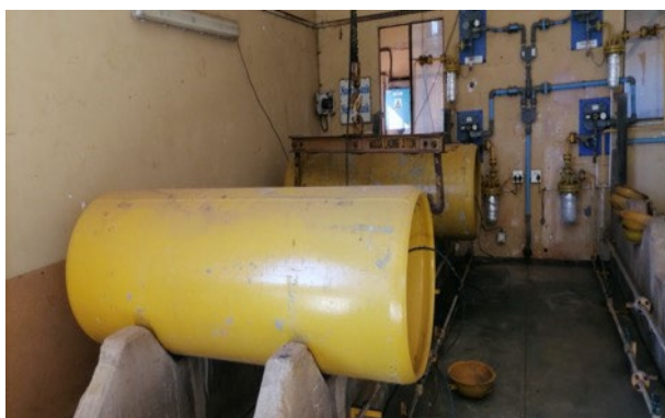
Figure 16: Empty tanks connected and not dosing due to lack of stock
