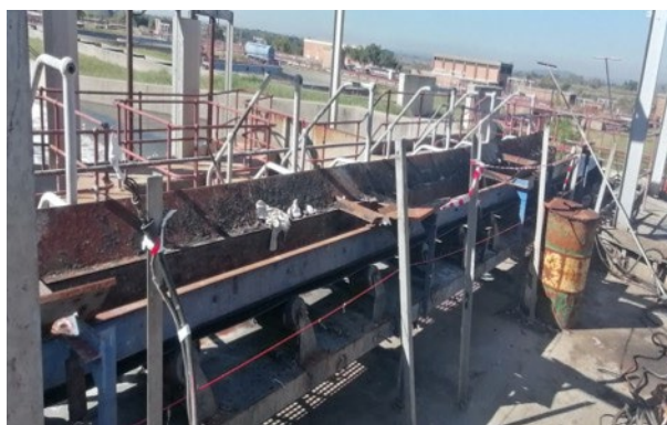
Figure 4: Poor condition of the conveyor belt
