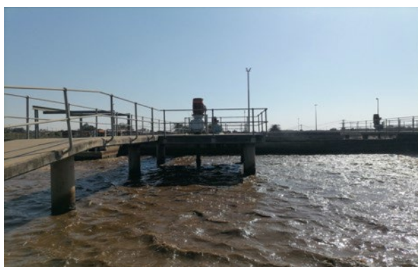
Figure 75: Aerator not working
