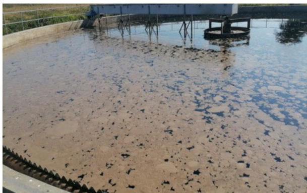
Figure 77: Excess scum formation due to faulty clarifier bridge motor
