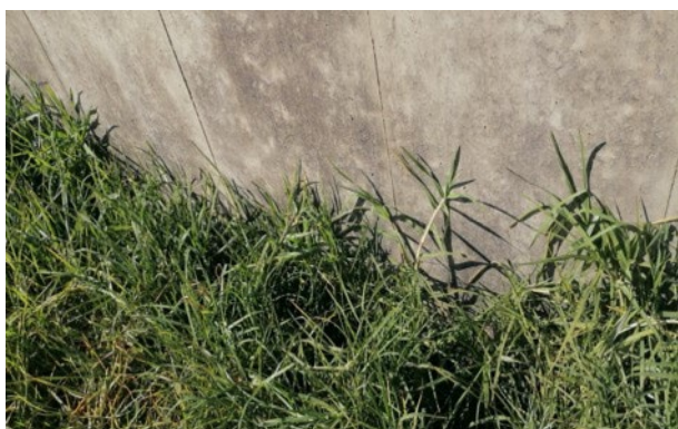
Figure 27: Poor conditions at some of the filter underdrains
