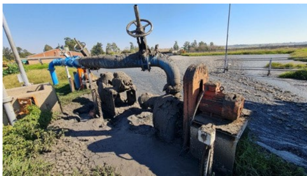
Figure 45: Sludge transfer pumps seen (One pump works whilst the other two are dysfunctional)
