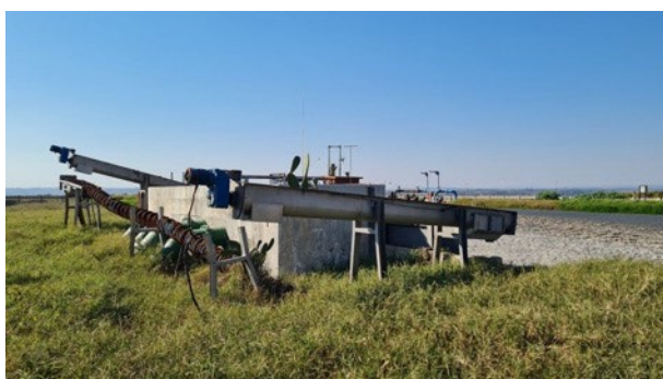
Figure 40: Northern sludge handling plant inlet works screens taken out and screw conveyor dysfunctional
