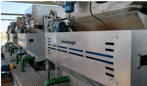
Figure 60: Sludge dewatering belt presses in a fair and working condition
