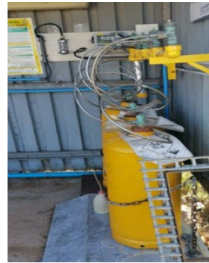
Figure 80: Dosing equipment without standby
