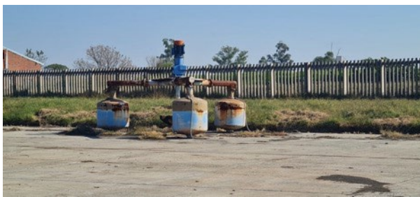
Figure 43: Floating surface aerators taken out
