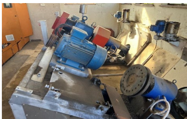
Figure 12: Typical condition of the RAS pumps, only one pump working
