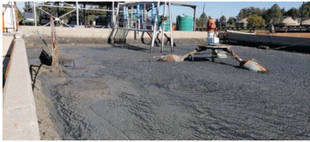
Figure 59: Floating surface aerators not working
