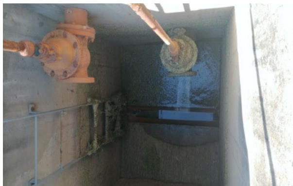
Figure 68: Sludge and scum withdrawal equipment in working condition
