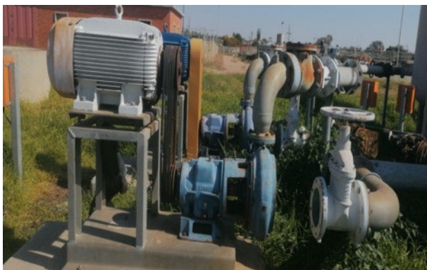
Figure 81: One of the DAF pumps not working
