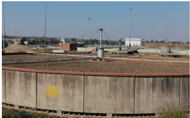
Figure 72: Filter out of commission due to excessive leaks
