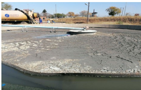
Figure 24: Excessive scum layer observed in all PSTs and a broken-down scrapper arm
