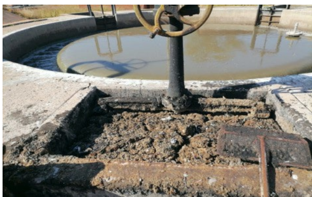
Figure 23: Excessive scum and grit accumulation in the division box inlet chamber
