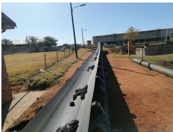
Figure 63: Dewatered sludge Conveyed to the Concrete Slap North of Rooiwal WWTW
