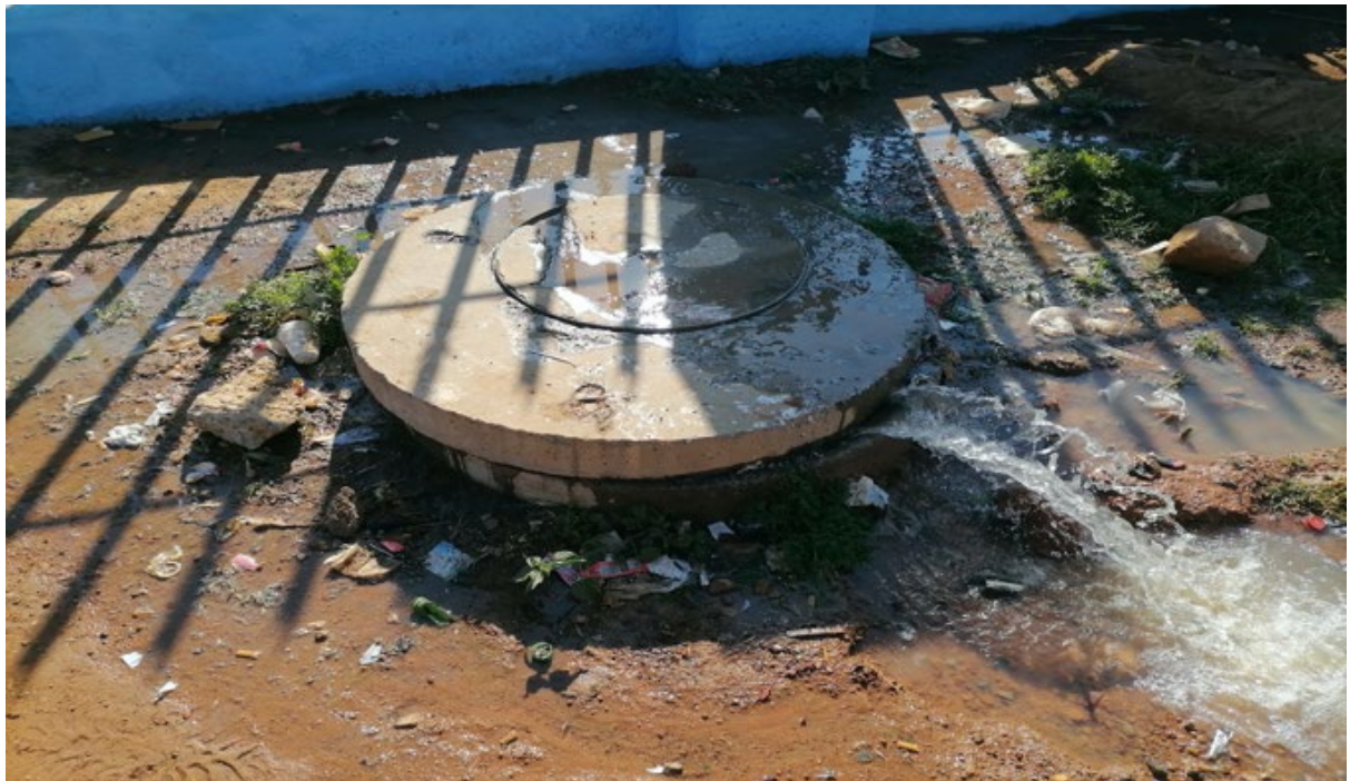
Figure 11: Overflowing sewage manhole
