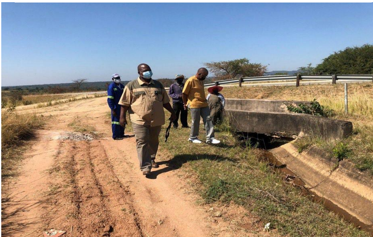
Figure 9. Major Challenges with unmaintained/damaged canals at New Forest Irrigation Scheme
