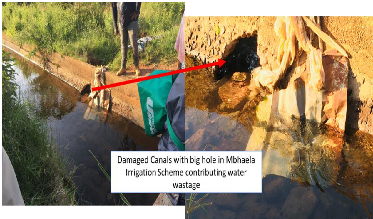
Figure 10. Damaged canals at Mbahela Irrigation Scheme
