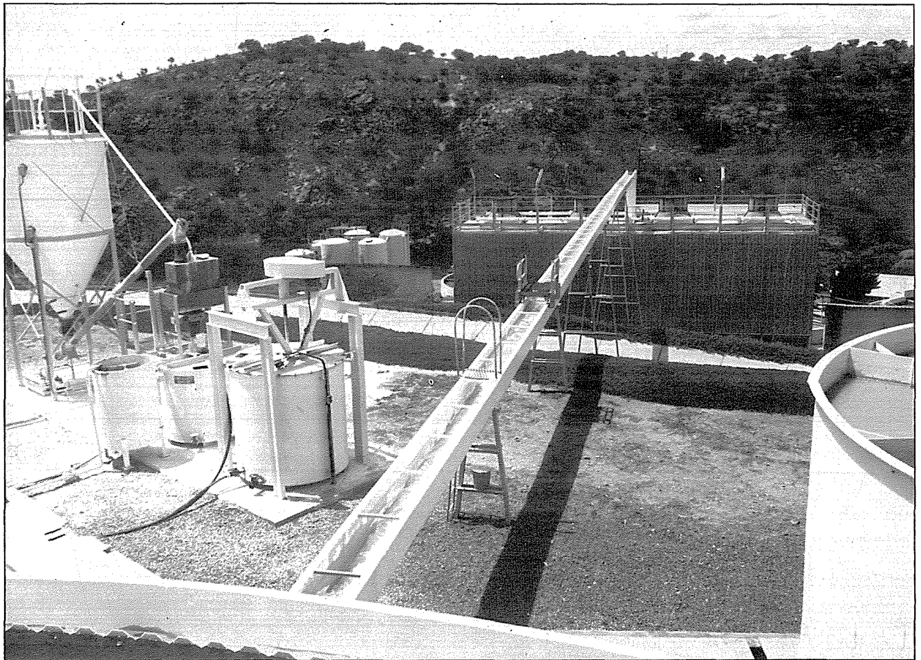
A part of the Windhoek Water Reclamation Plant which continues to play an important role in the city's water supply. The conduit (centre) leads from the primary sedimentation tank to the ammonia stripping tower. To the left (in the far background) the activated carbon columns, and on the extreme left the lime container may be seen.
