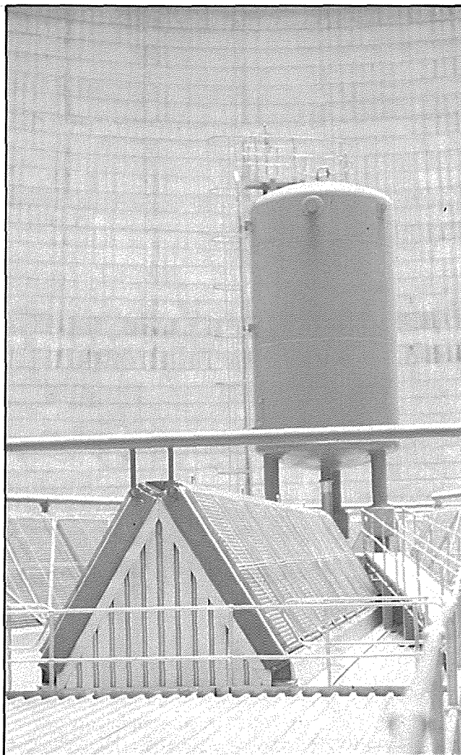
A typical dry cooling element in the foreground in a cooling tower at a power station
