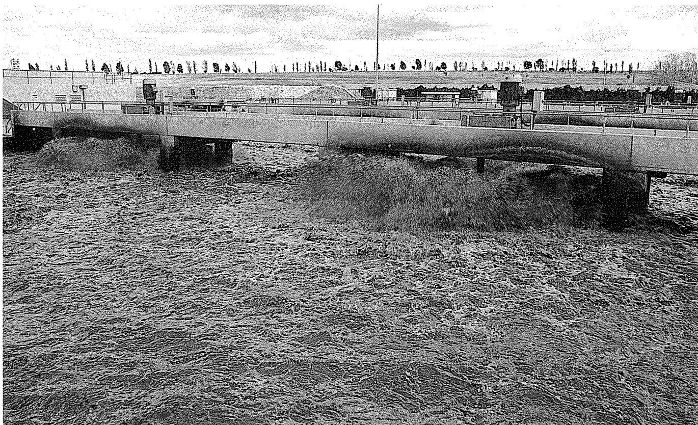
Surface aerators at the Northern Sewage Purification Works, Johannesburg, where research on biological phosphate removal is being carried out.
