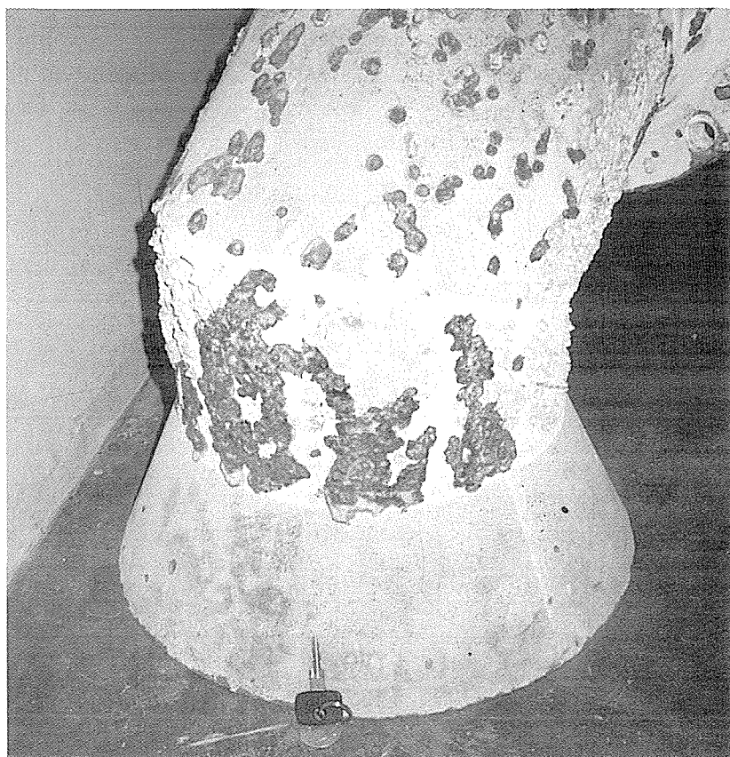
A typical example of biocorrosion on a pipe immersed in water.
