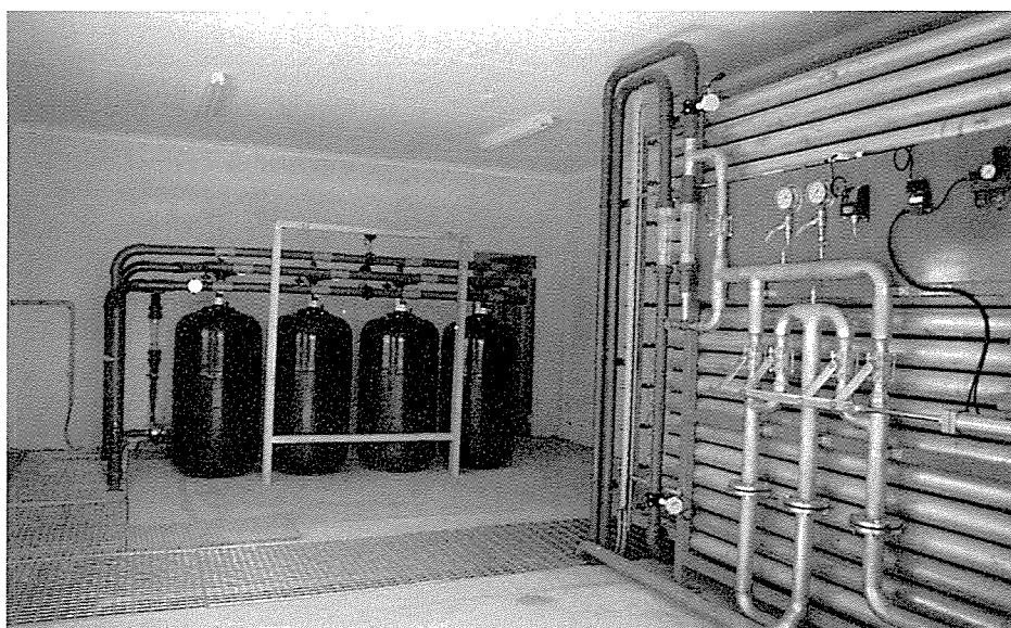
The Bitterfontein tubular reverse osmosis plant for producing potable water.
