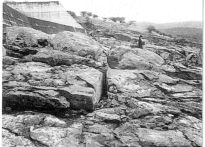
Erosion downstream of the concrete structure at the Goedertrouw Dam
