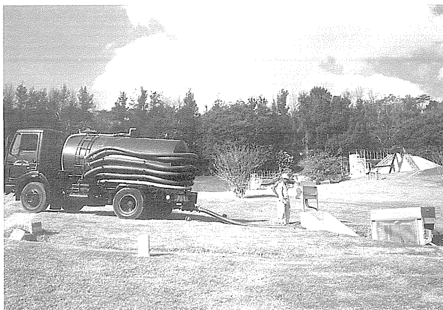
Feeding concentrated dye effluent into the anaerobic digesters at the Umbilo Sewage Purification Works at Pinetown, Durban. The digester is in the background.
