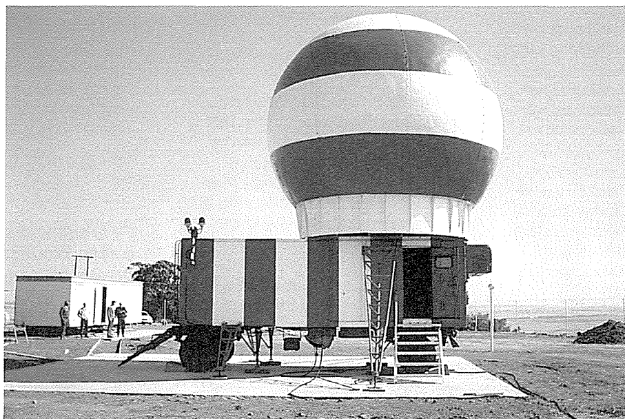
The new double wavelength (S- and X-band) radar system which has been installed at Bethlehem in the Free State.
