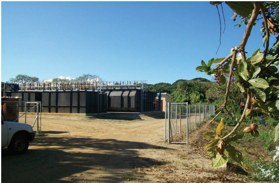
Figure 9: The Melville Wastewater Treatment Works
