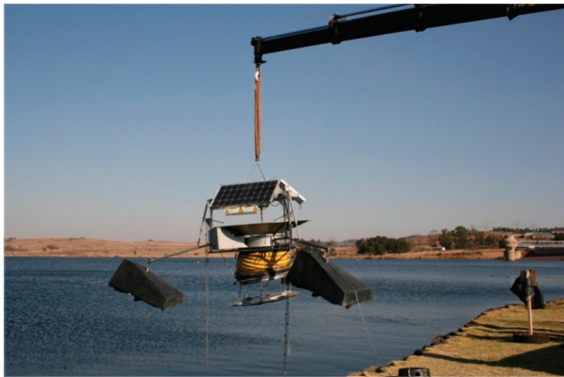
Figure 9 Deployment of a SolarBee® laminar flow pumping unit in Rietvlei Dam during 2008
