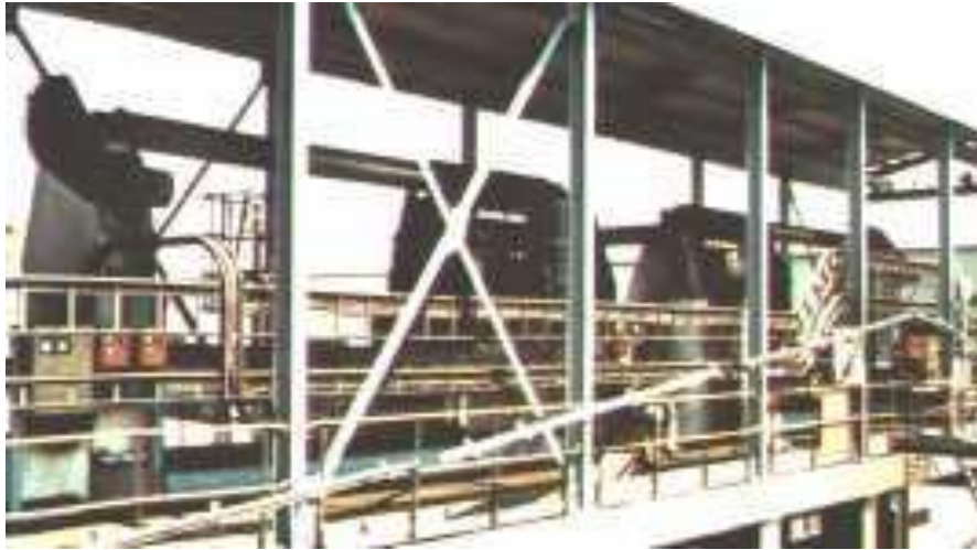
Figure 57 - Shriver Filter Press at Middelburg South Plant
