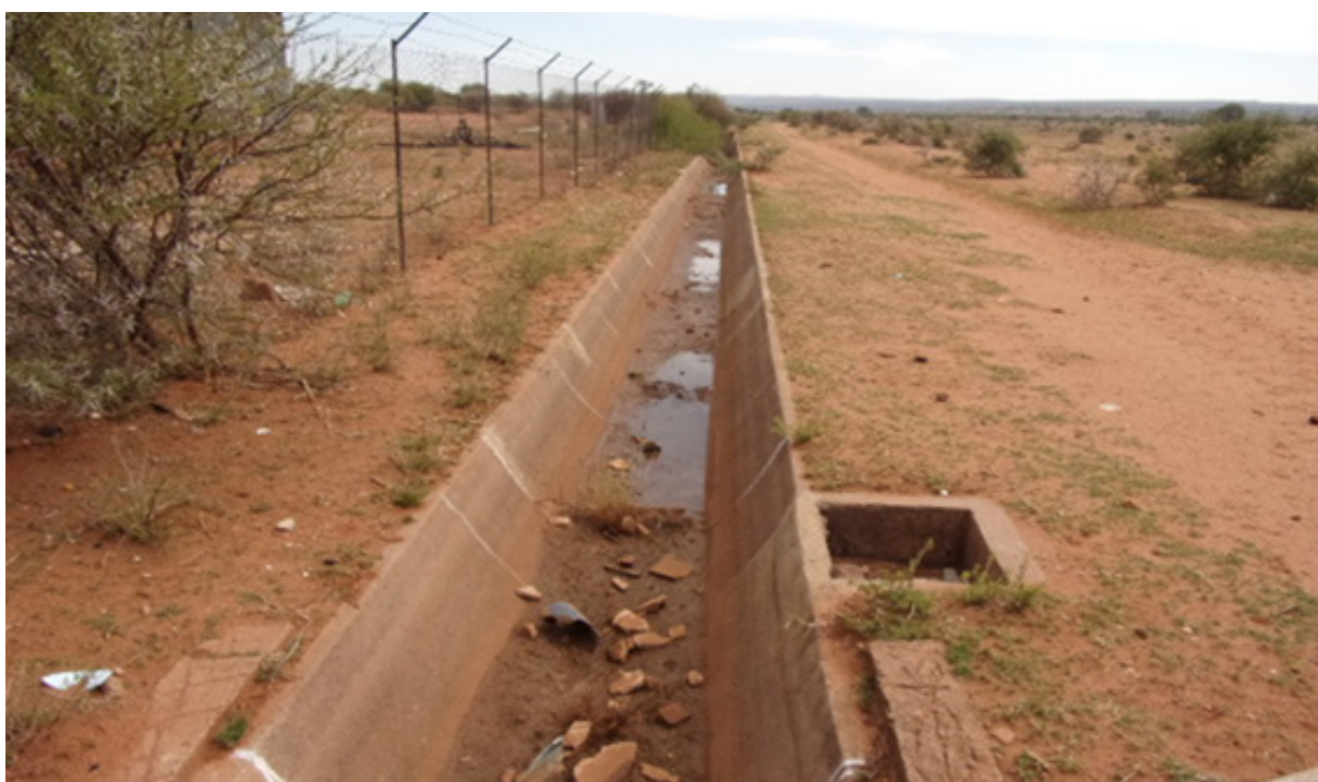
Figure 2. State of irrigation canals in most irrigation schemes
