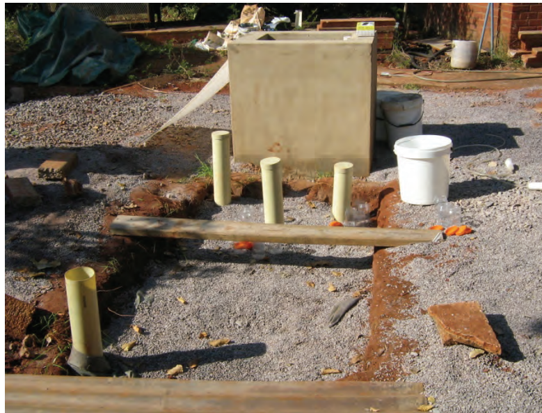
Figure 7.7: Combination of mulch tower and sub-surface resorption bed, including embedded infiltration zone and surrounding gravel filter. Note access points for sampling.
