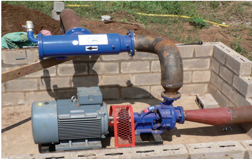
Figure 13. Electric motor with covered coupling, single stage pump and outlet through filter
