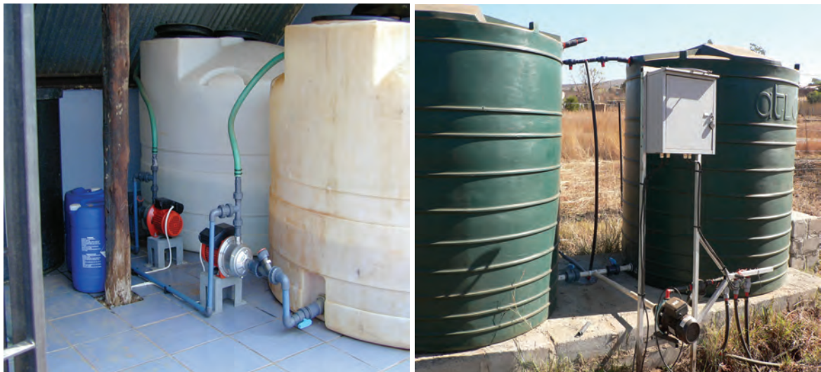
Figure 3. Tank A and B with various fertiliser mixtures fitted with fertilizer pumps
