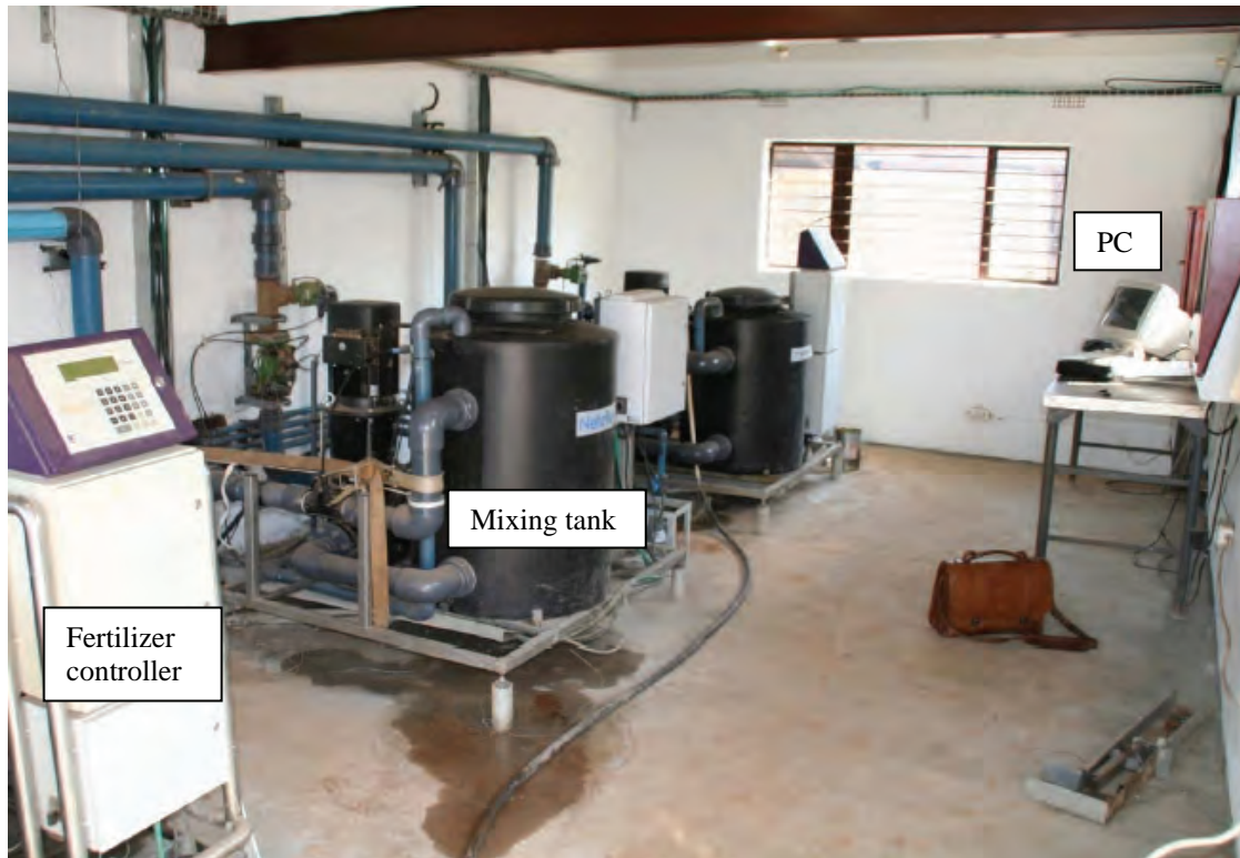
Figure 14. Fertilizer control room
