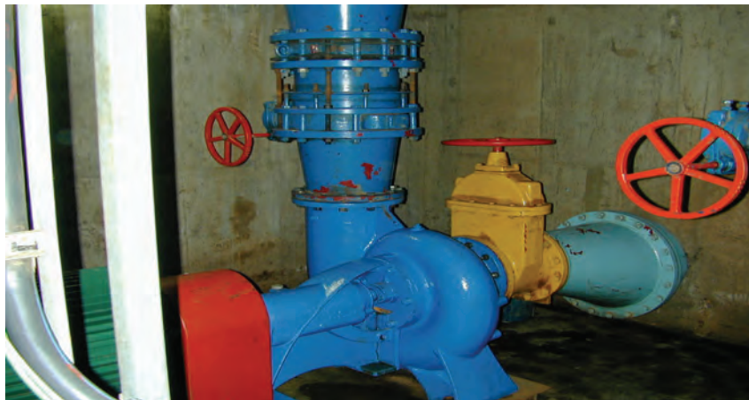
Figure 20. Pump outlet with main valve (top) and shut off
