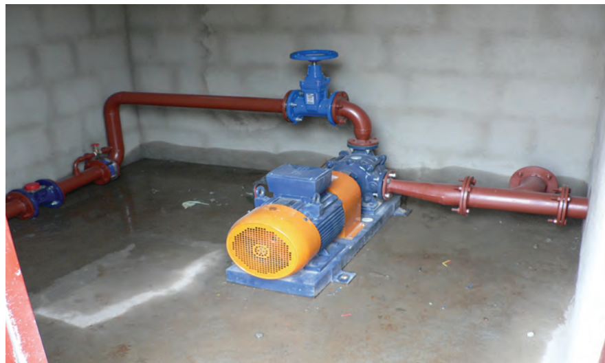
Figure 14. Motor and pump, inlet [right], outlet with main valve, non return valve with bypass and water meter
