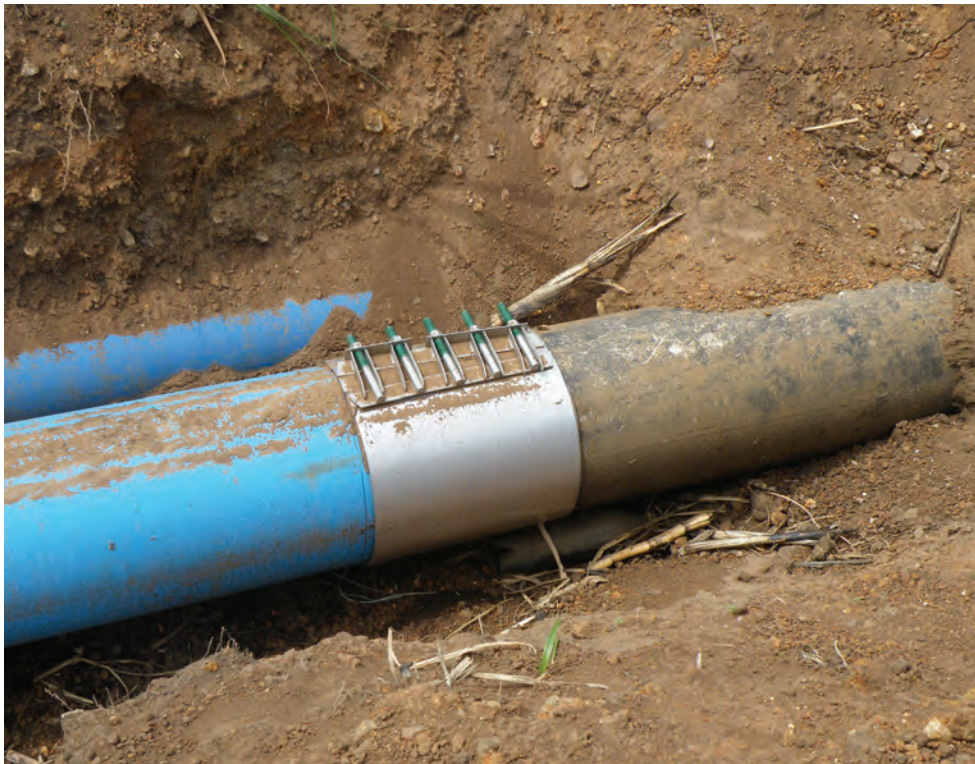
Figure 30. PVC pipe connected to asbestos cement (AC) pipe
