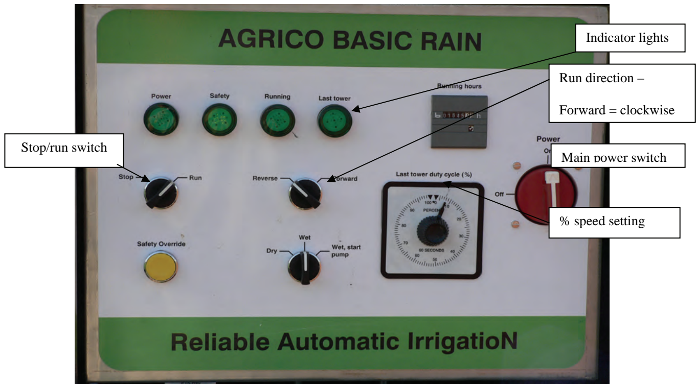
Figure 27. Centre pivot control panel
