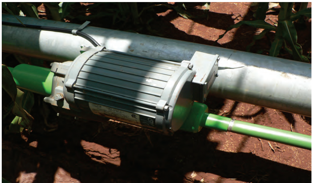
Figure 25. Electric motor and drive shafts
