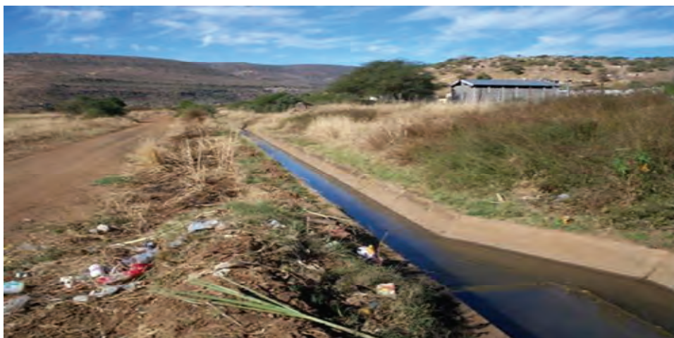
Figure 1. Debris that have been removed from a canal at Tugela Ferry
