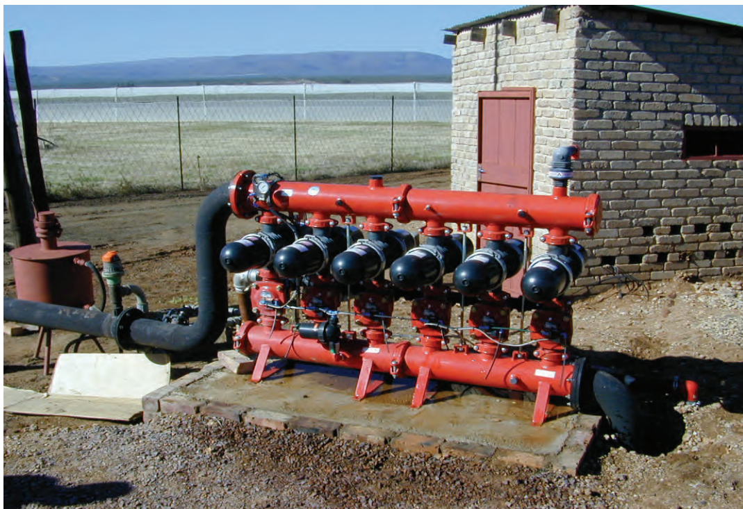
Figure 25. Automatic flushing disc filters
