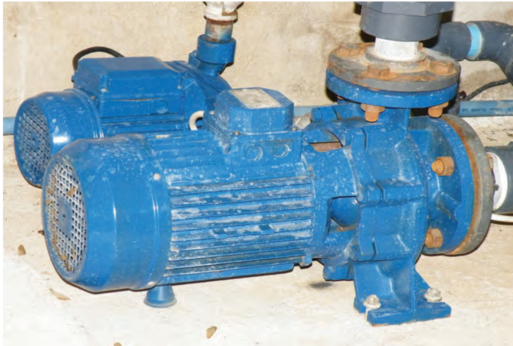
Figure 12. Close coupled pump and motor
