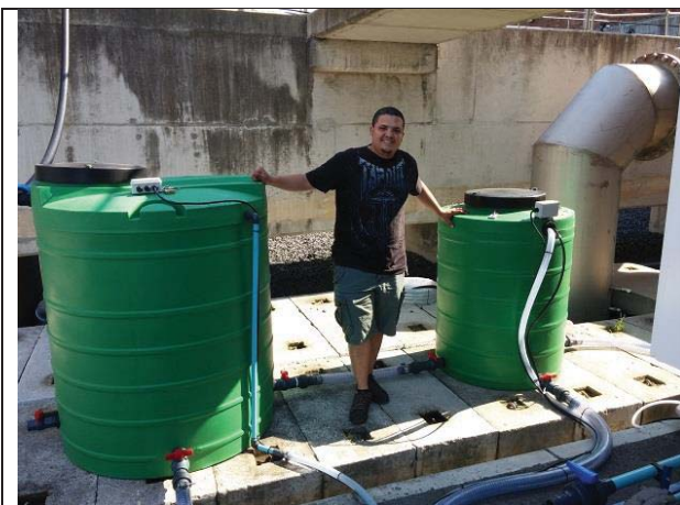
bioreactor (left) and membrane tank (right)
