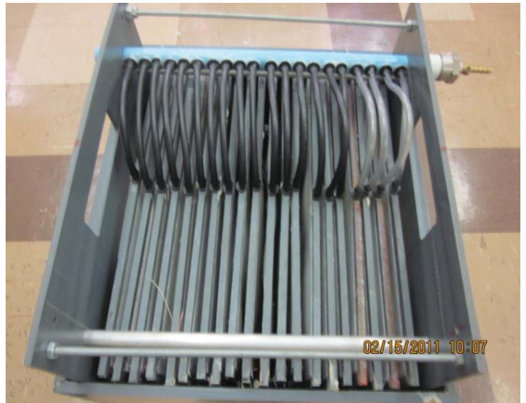
Permeate off-takes on panels
