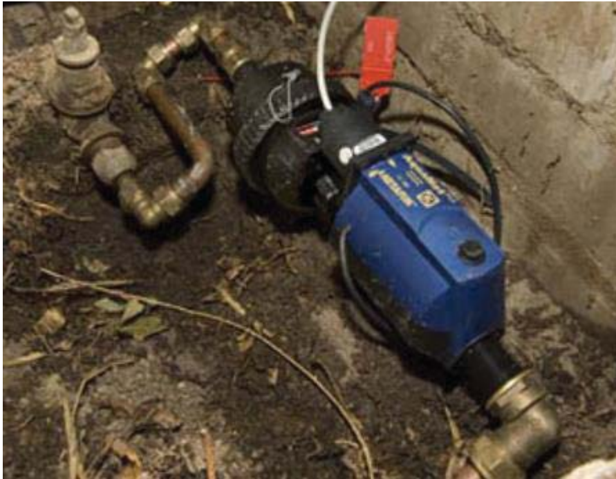
Figure 11: The set-up of a water meter and a water management device (Pollark, 2009)
