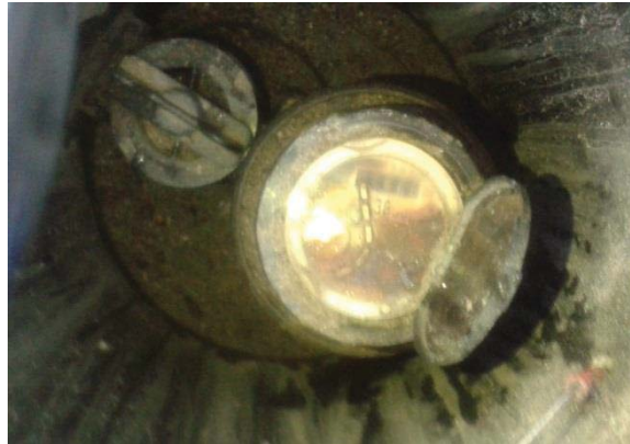
Figure 59: Obscured water meter screen
