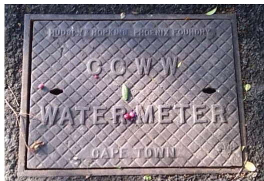
Figure 60: Heavy metallic lid covering the meter box
