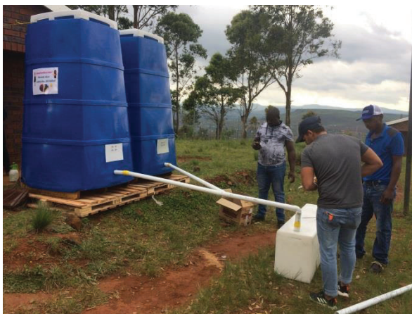
Figure 37: 200-litre storage tank was placed below the outlet from the urinal units, to enable gravity flow of urine into the tank and storage
