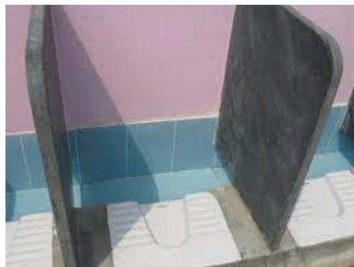
Figure 23: The squatting urinal design, including a ceramic squat pan with raised foot spaces to reduce splashing, and a tiled channel for discharge of urine
