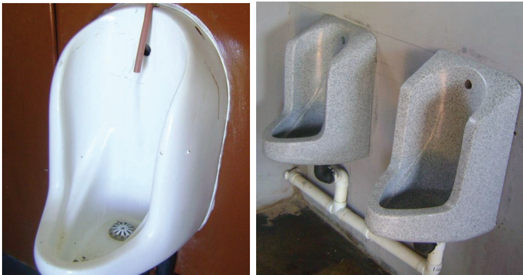
Figure 6: Typical wall-mounted ceramic urinal at Laduma High School (left) and plastic urinals at Shayabantu High School (right)
