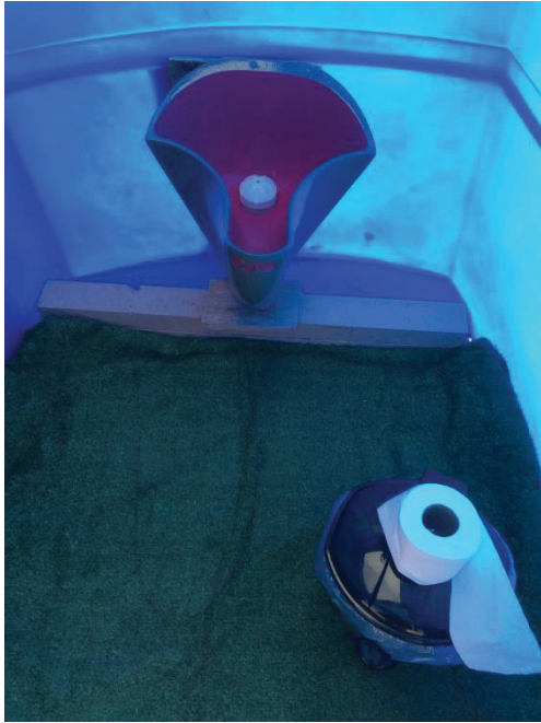
Figure 35: Weestand installed in the toilet hut; both toilet huts were equipped with a bin for toilet paper
