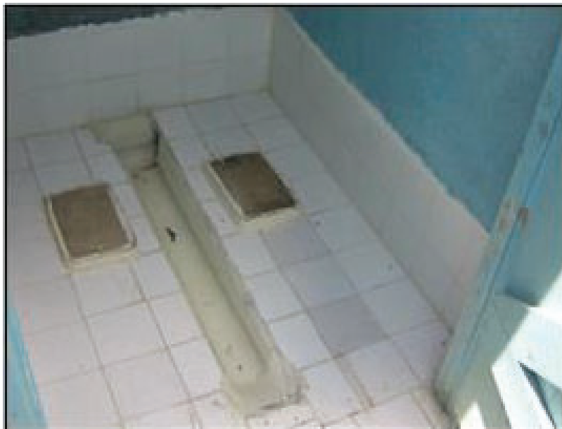
Figure 18: Urinal with tile floors, installed at Atono Primary, Kenya; the use of tile for the floors makes cleaning simpler
