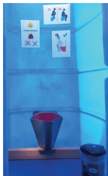
Figure 34: Toilet huts decorated with necessary messaging to ensure that the users used the urinals correctly
