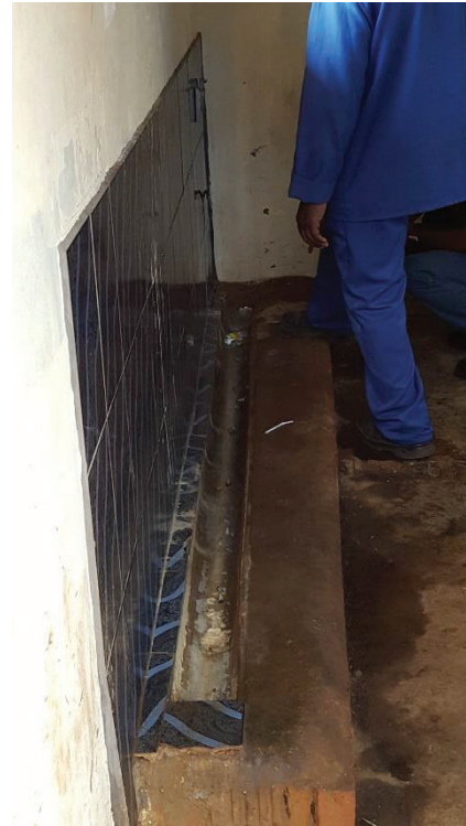
Figure 4: Phayiphini Urinal 2 – This urinal in another block of boys' toilets at the school is slightly better than Urinal 1, in that the tile work extends to the floor around the urinal and that a gutter has been used to create a drain that is more water-resistant, providing better drainage. However, the area in front of the urinal is again not painted with water-resistant epoxy, leading to the same odour issues as in Urinal 1. As can be seen in the photo, cracks and edges in the urinal also make it difficult to clean.
