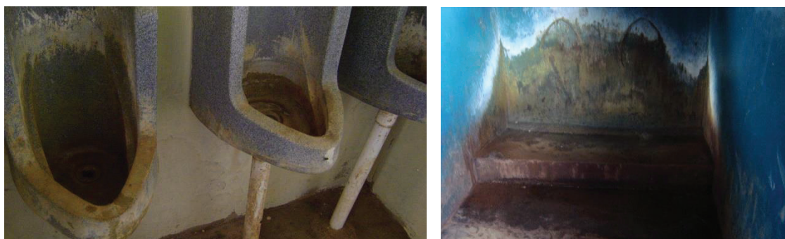
Figure 26: Unsanitary impact of scaling from urine and improper cleaning regime observed in Vezokuhle Primary School (left) and Imbubu Primary School (right)
