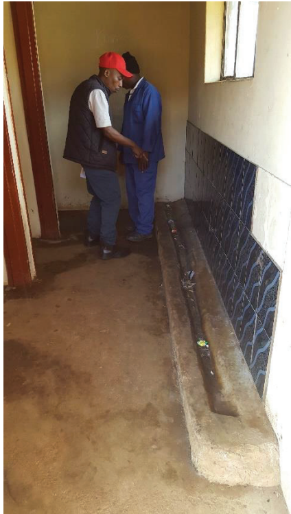
Figure 3: Phayiphini Urinal 1 – The design of this urinal uses tiles to protect the wall. However, water-resistant material, such as epoxy, has not been applied to the drain and surrounding area, which has led to excesses of urine soaking into the concrete, creating unpleasant odours. In addition, the drain is shallow and not properly sloped, leading to insufficient drainage.
