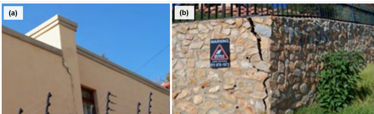
Figure 4-1 Cracking and failing of walls and retaining wall due to leaking pipeline upstream (photograph by Dippenaar).
