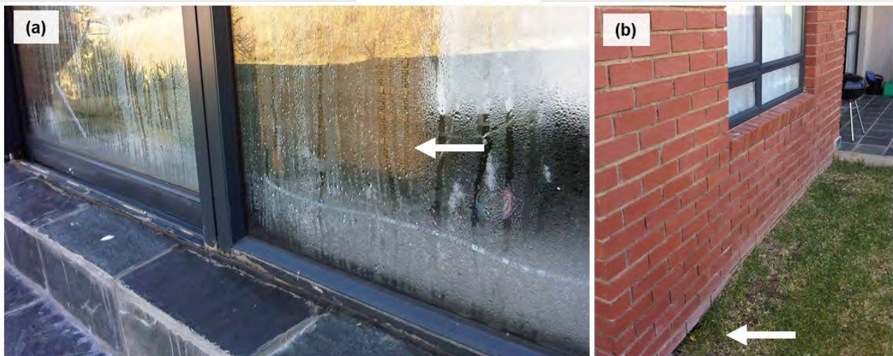
Figure 4-5 Water from golf course irrigation that caused (a) damp to rise inside the house and (b) erosion of soil under the house (photograph by Dippenaar).
