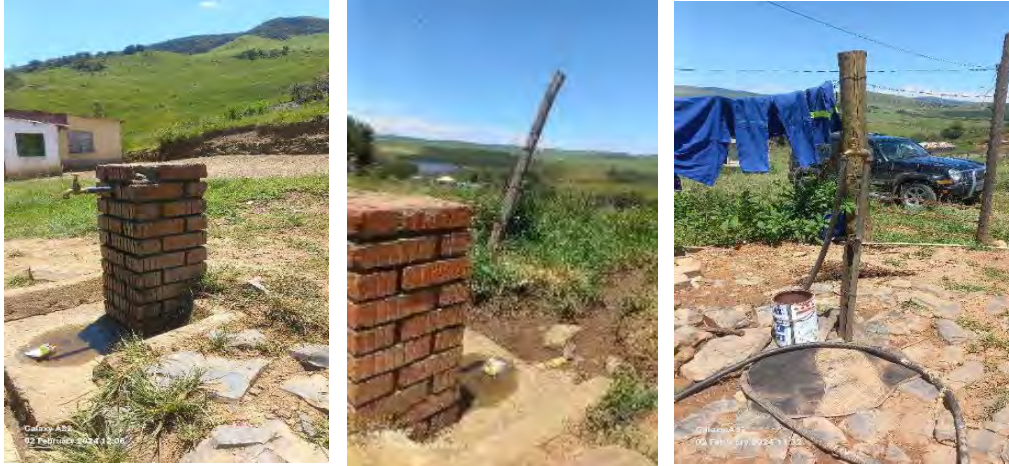
Figure 29: Pictures showing communal standpipes set up by Mvula Trust and a private yard connection subsequently undertaken by some of the households themselves (illegal connections)
