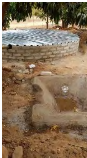
The silt trap for a 25 000l underground tank to reduce silt load of stored
