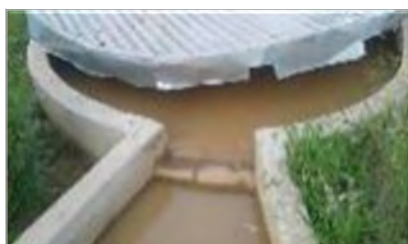
An example of an underground tank (18m 3 ), with a removable metal roof
