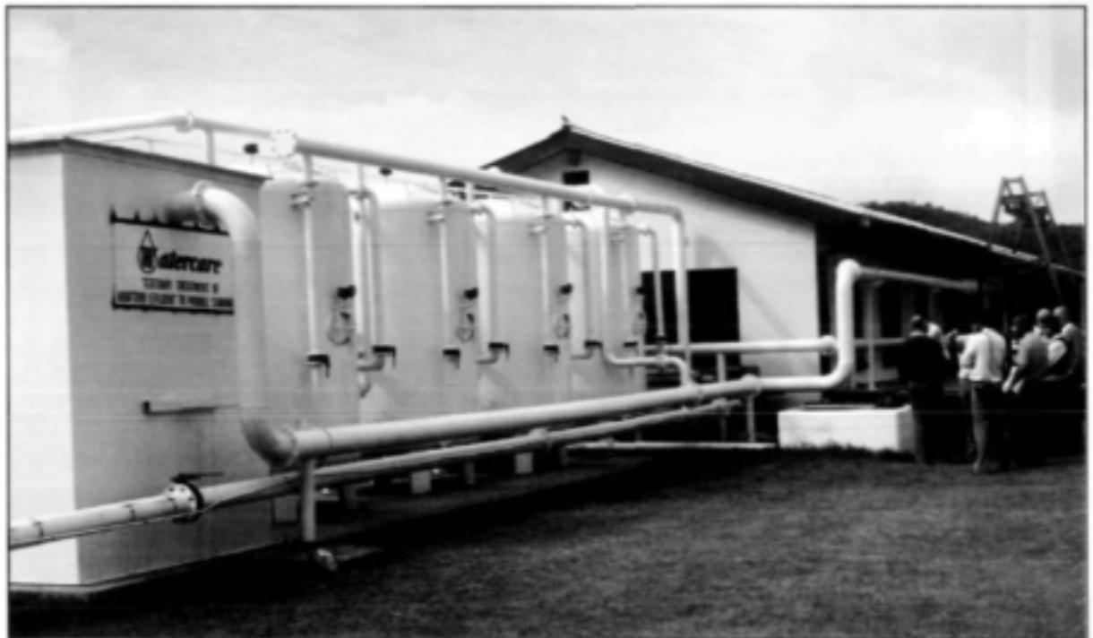
Figure 16: General view of package treatment plant
