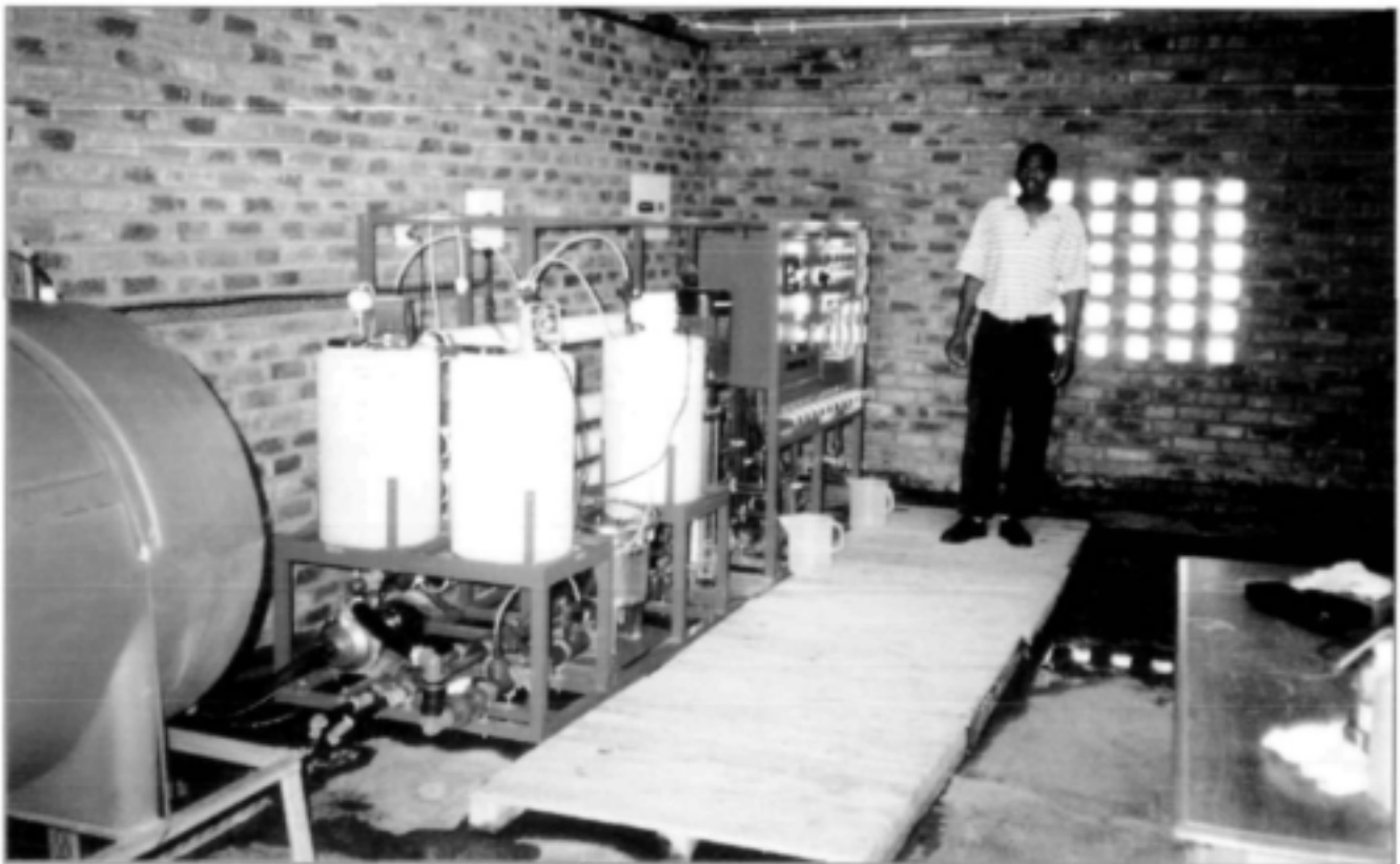
Figure 18: Small-scale RO plant
