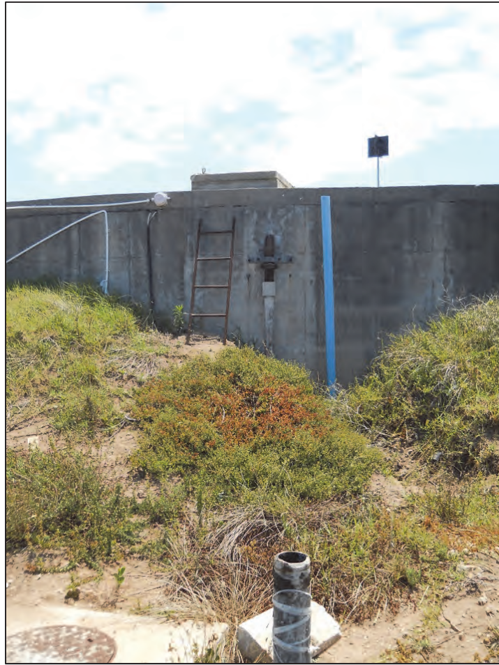
Figure 6-6: Fraaiuitsig Reservoir inlet
