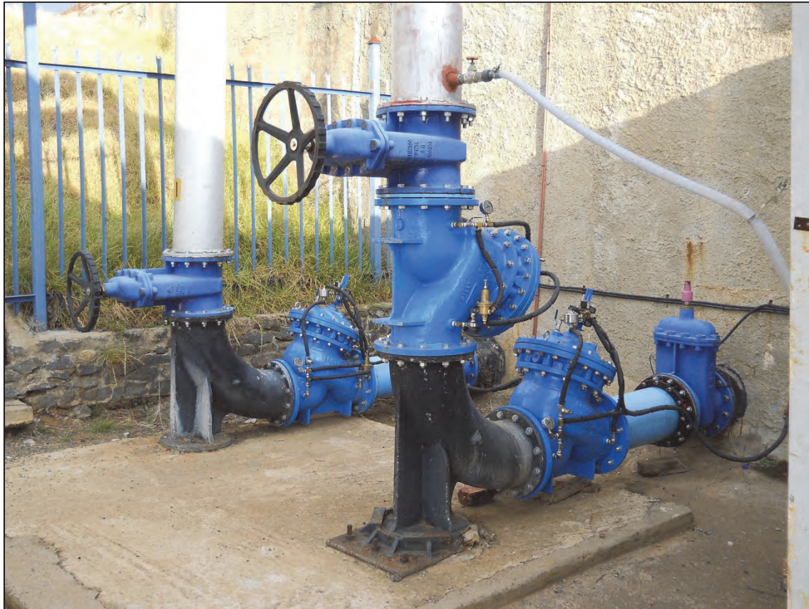
Figure 4-11: Refurbished pressure reducing valves on Branch 1 and 2
