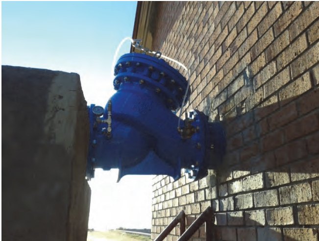
Figure 4-52: Pressure/flow control valve regulating supply to turbine room
