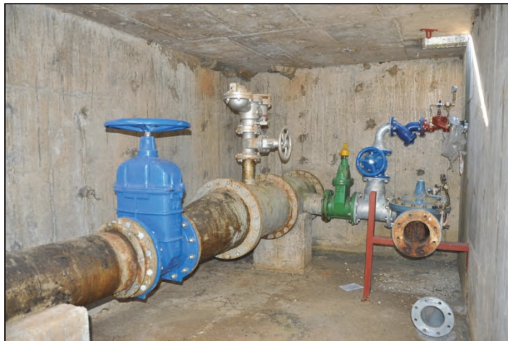
Figure 6-35: Chamber at Sandile WTW
