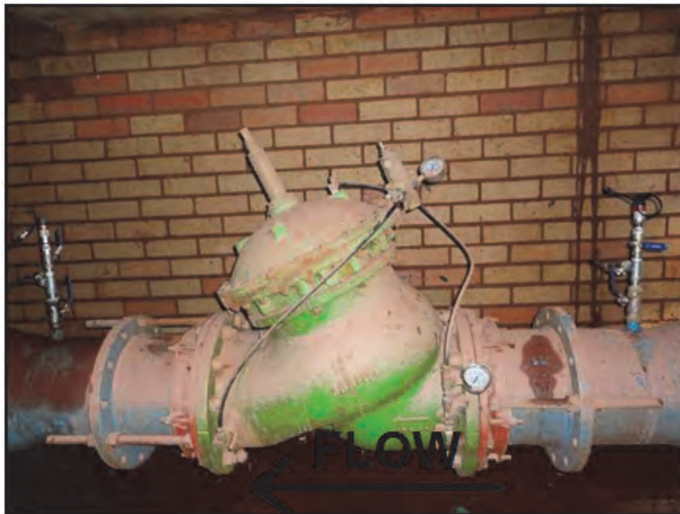
Figure 3-16: Pressure transducers fitted either side of the PRV
