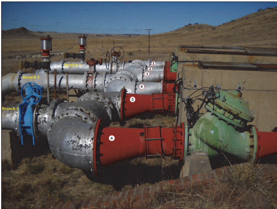
Figure 4-3: Inlet manifold at Uitkijk Reservoir
