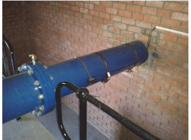
Figure 4-53: Pipeline upstream of turbine with ultrasonic flow meter
