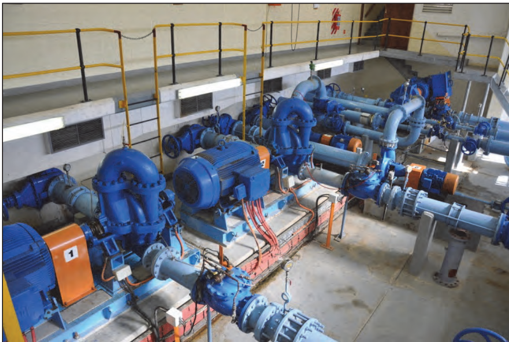
Figure 6-30: Sandile pump station
