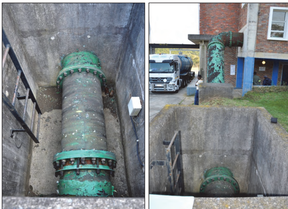
Figure 6-25: Chamber upstream of the Nahoon WTW
