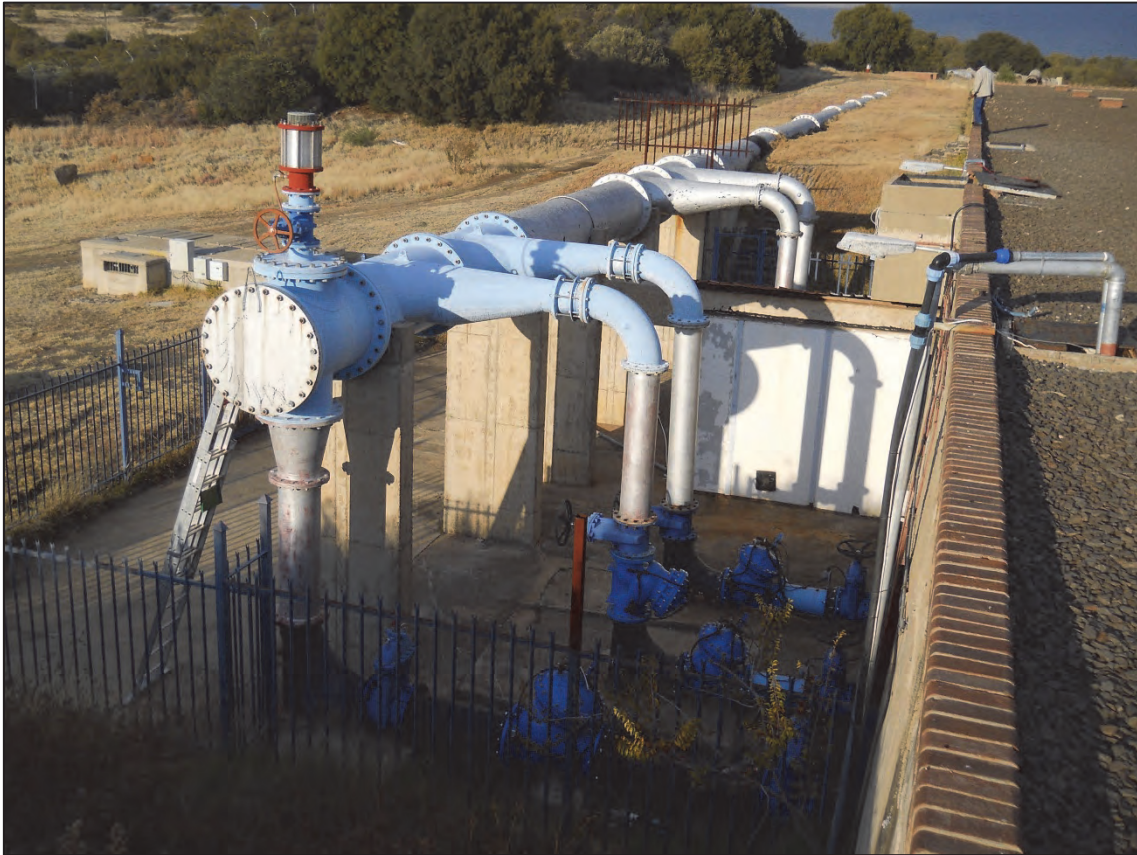
Figure 4-10: Refurbished pressure control station at Brandkop Reservoir
