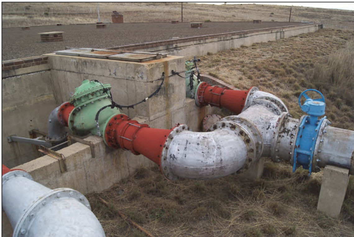
Figure 4-5: Control valves (branch 3) at Uitkijk Reservoir inlet
