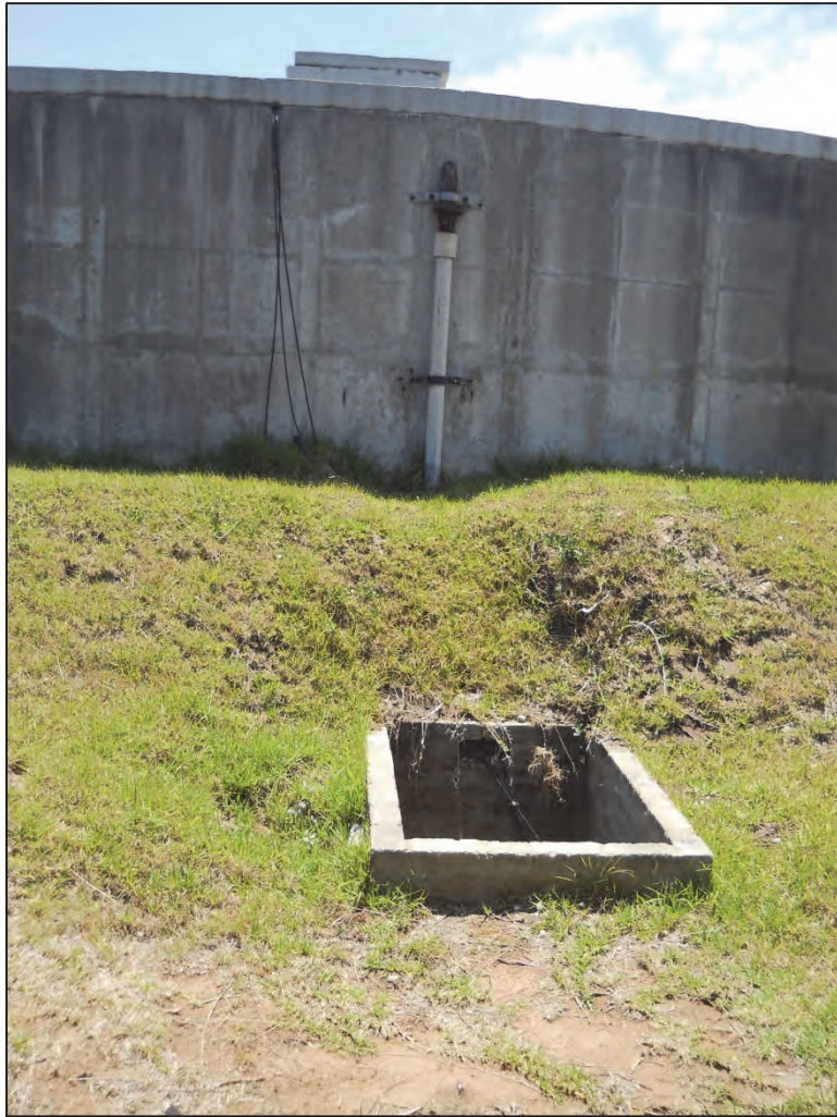
Figure 6-7: Tergniet Reservoir inlet
