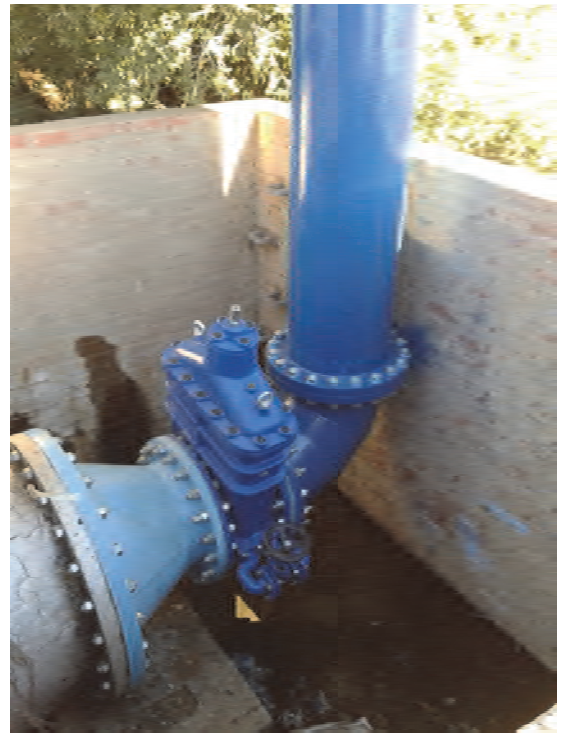
Figure 4-49: off-take connected to isolating valve
