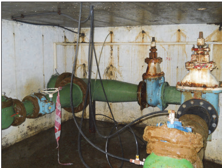
Figure 5-11: Cross connections in the PRS chamber
