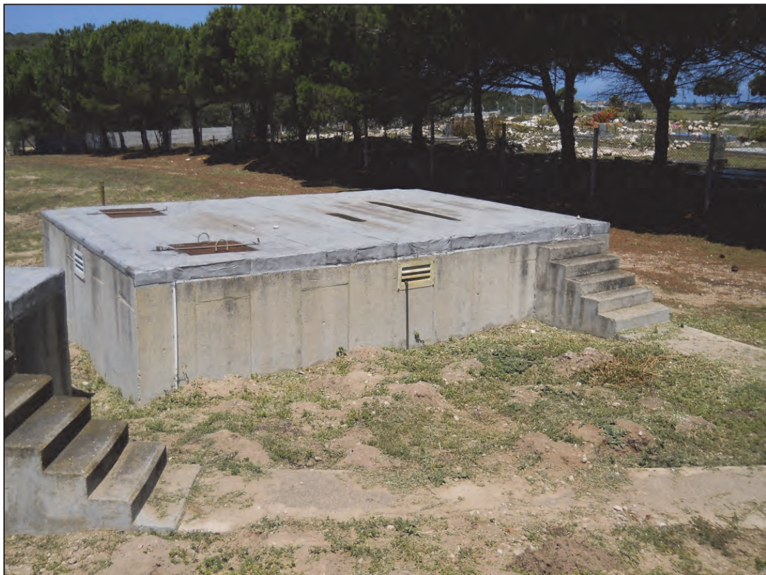
Figure 6-15: PRS on bulk supply pipeline from Wolwedans Dam
