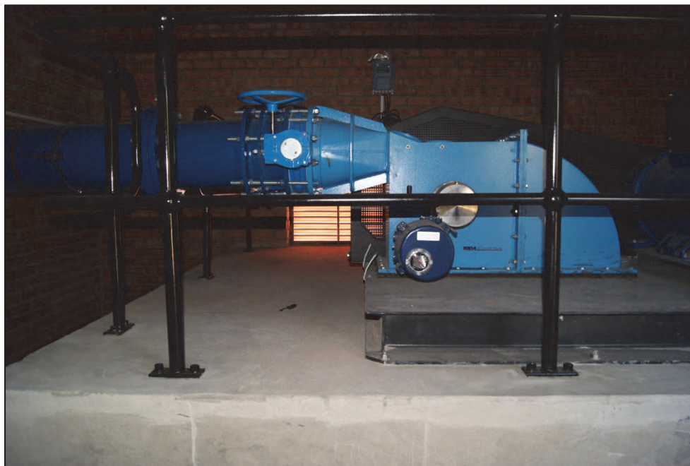
Figure vii: Brandkop hydropower installation
