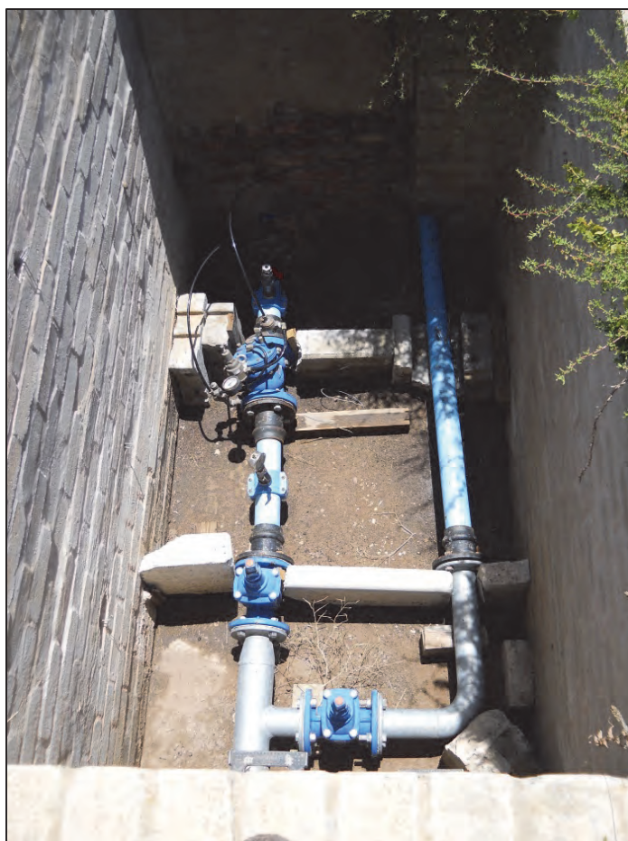
Figure 6-4: Pressure reducing station (Fraaiuitsig Reservoir)
