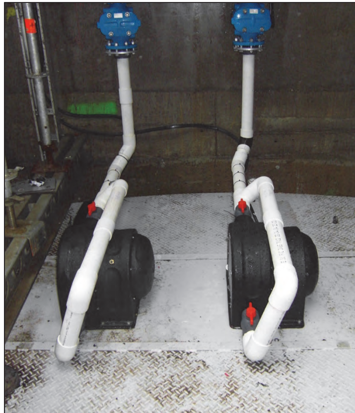
Figure 5-3: Example of Powerspout turbines installed in parallel
