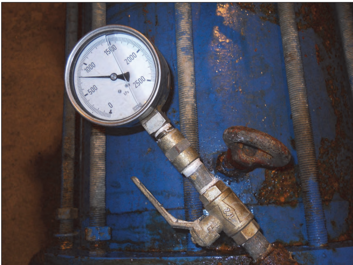
Figure 6-17: Upstream pressure at PRS on bulk pipeline from Wolwedans Dam
