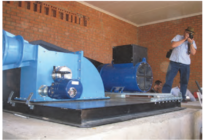
Figure 4-55: Turbine and generator in position
