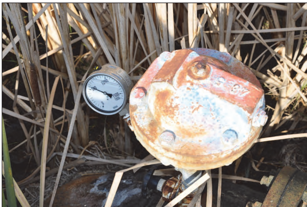
Figure 6-33: Control valve upstream of Sandile balancing tank
