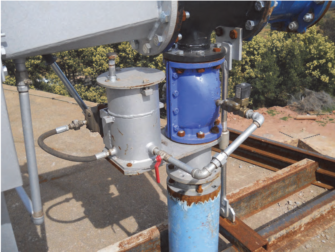
Figure 3-64: Emergency pinch valve (discharging into reservoir)
