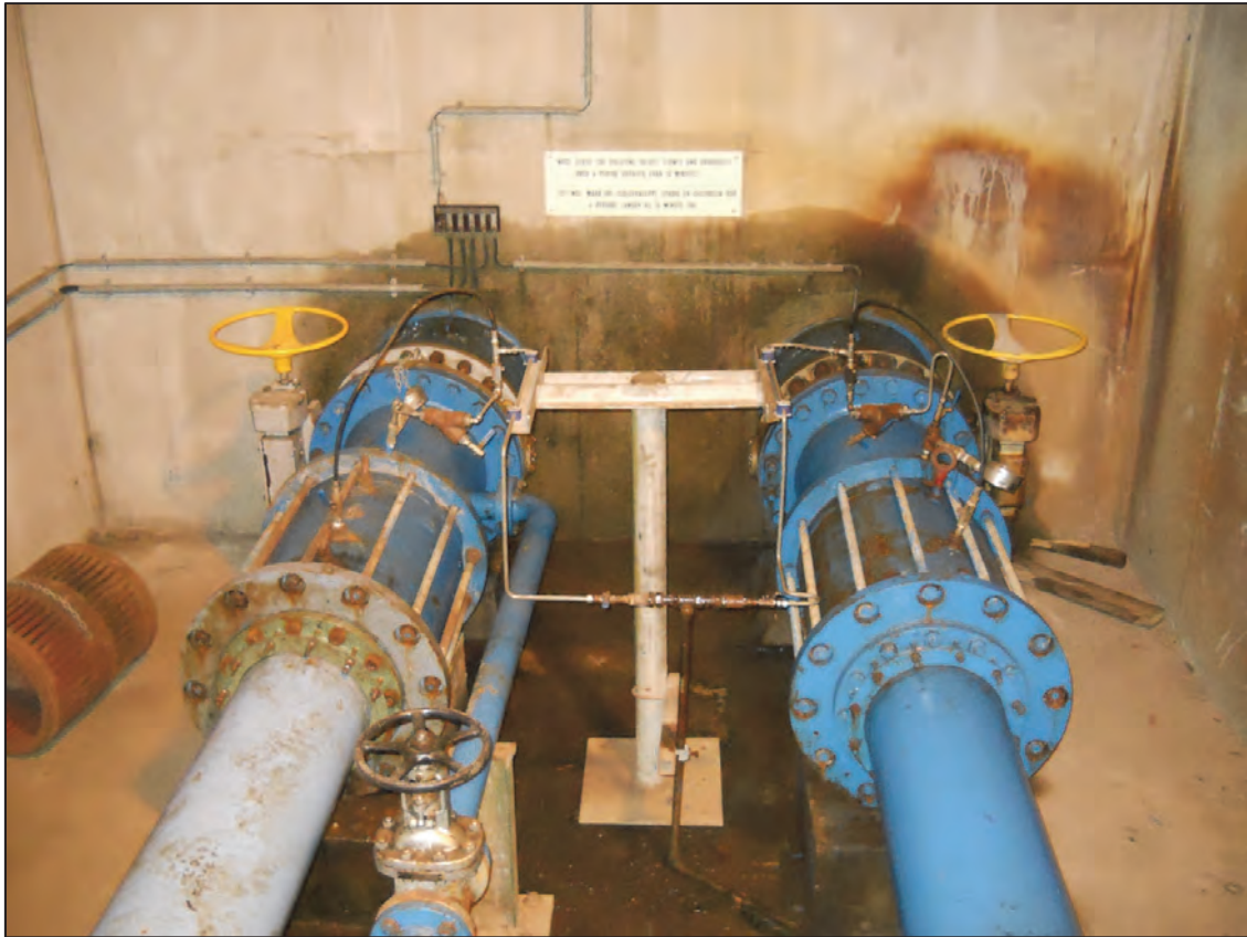
Figure 6-16: Two 300 mm Flexflo pressure control valves in PRS on bulk pipeline from Wolwedans Dam
