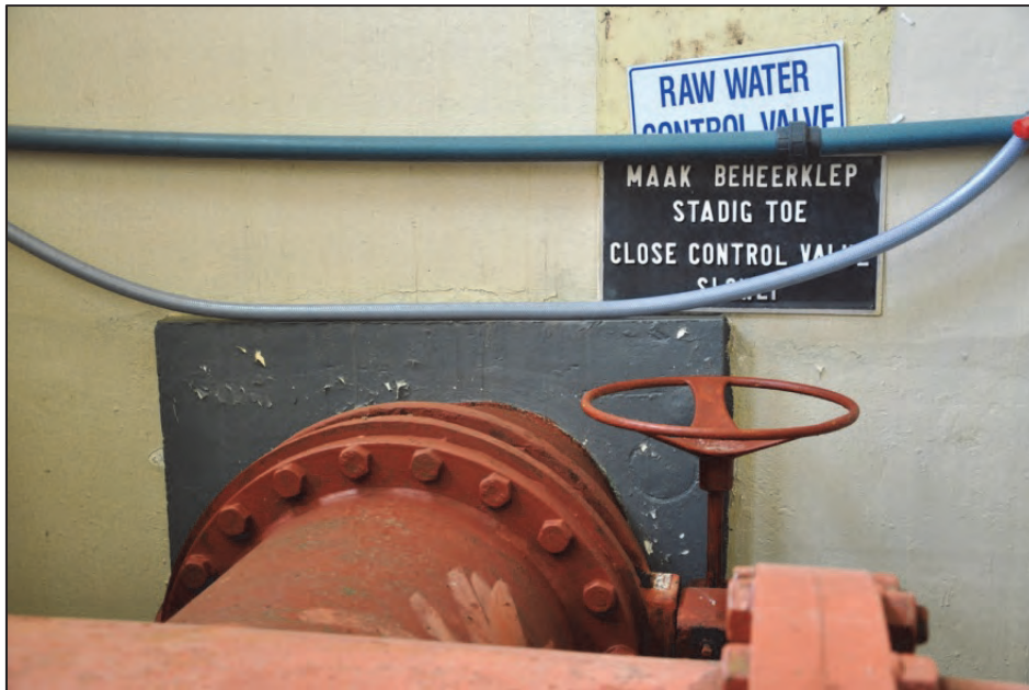
Figure 6-31: Control valve upstream of Nahoon inlet chamber
