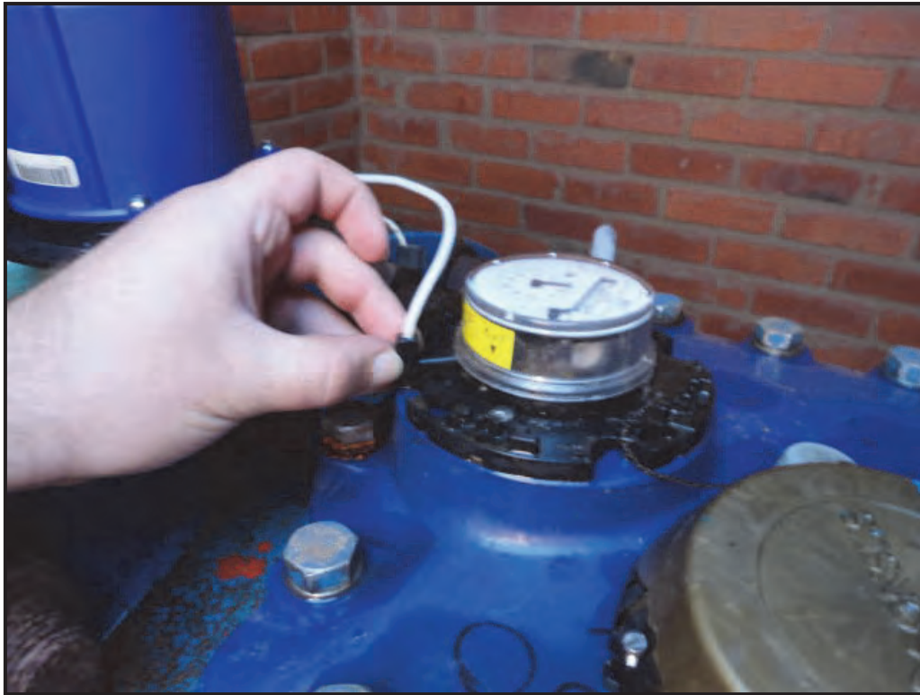
Figure 3-22: Connection of GSM wireless logger to flow meter
