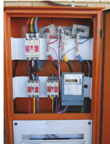
Figure 4-45: Recording electricity consumption of the Bloemwater head office
