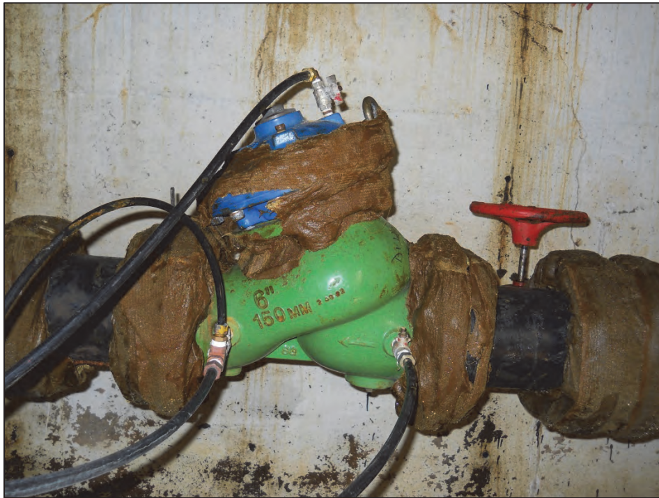
Figure 5-10: Pressure Reducing Valve (PRV)
