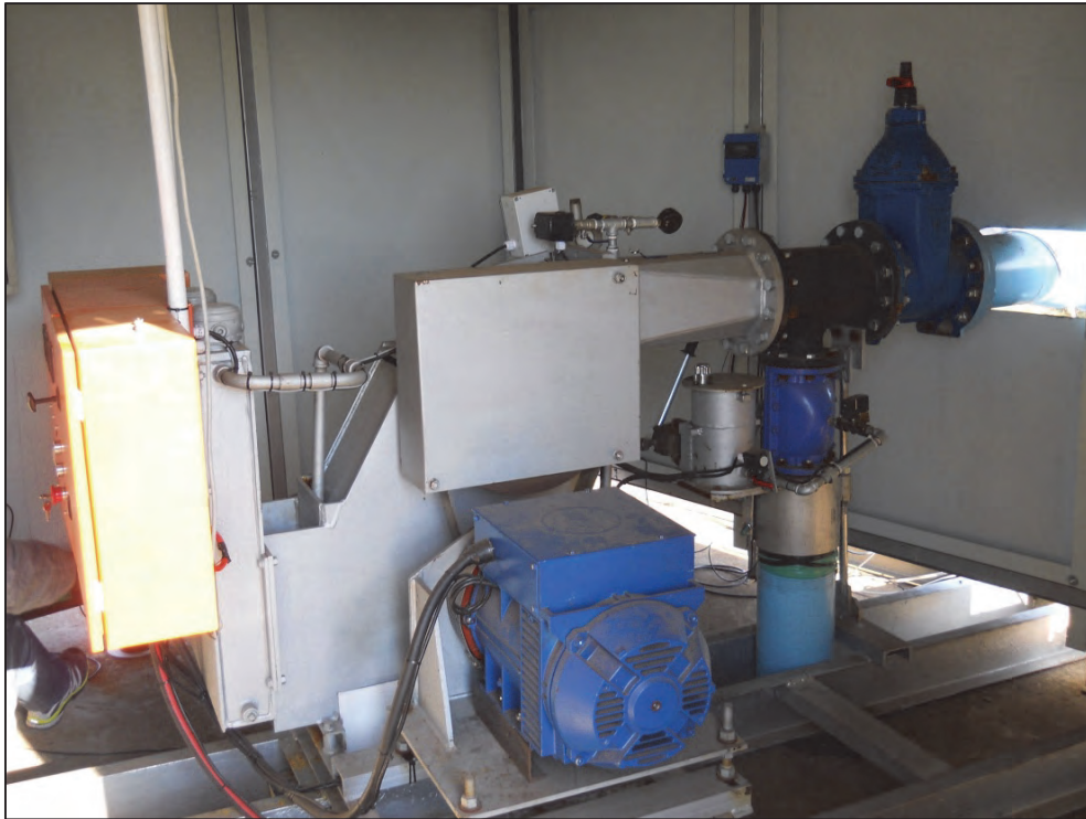
Figure vi: Pierre van Ryneveld hydropower installation
