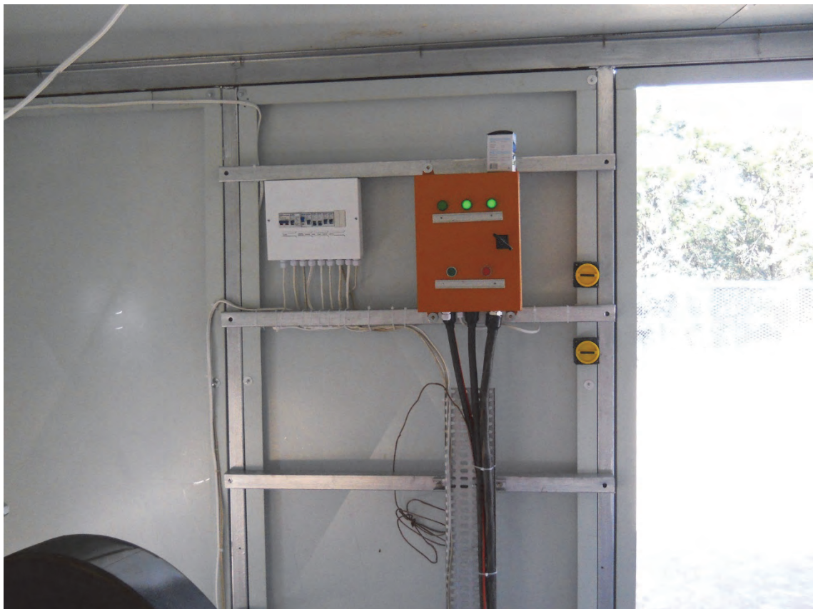
Figure 3-67: Electrical switch over (grid power or hydropower)
