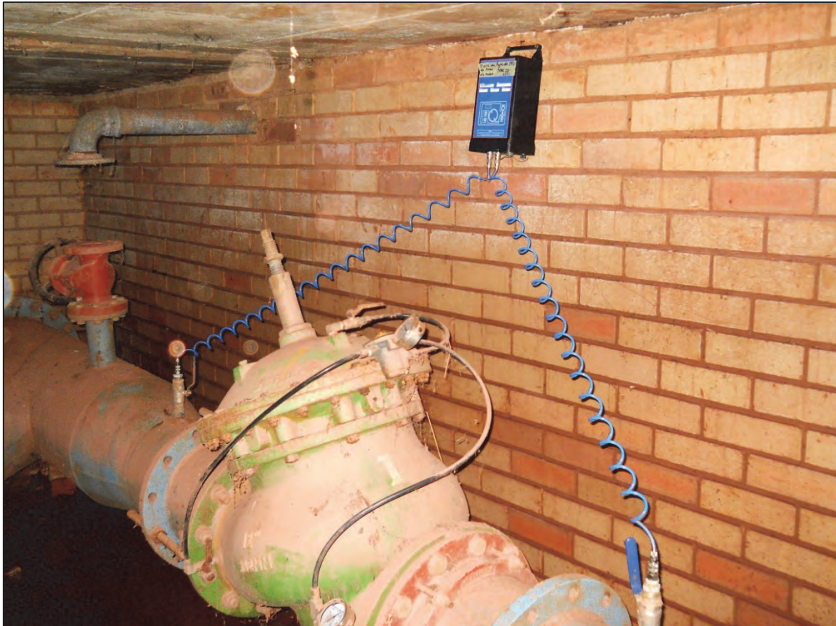
Figure 3-35: Pressure measurement at Pierre van Ryneveld pressure-reducing station
