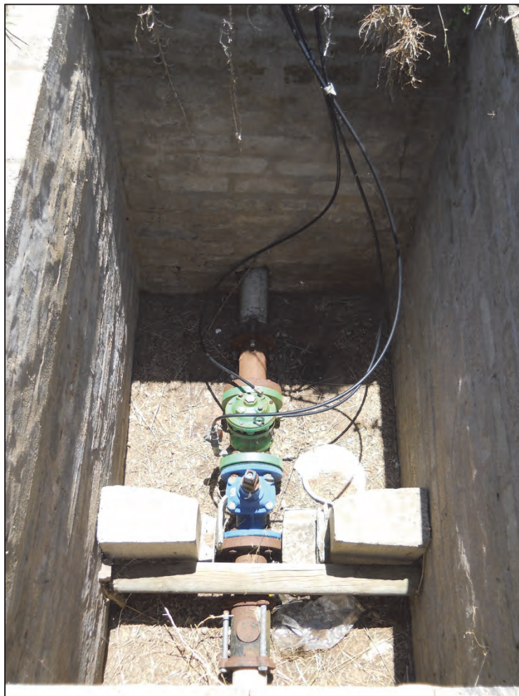
Figure 6-9: Tergniet Pressure Reducing Station
