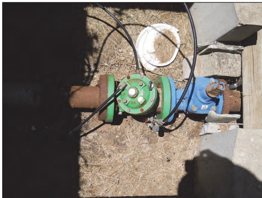
Figure 6-8: Pressure reducing valve upstream of reservoir inlet
