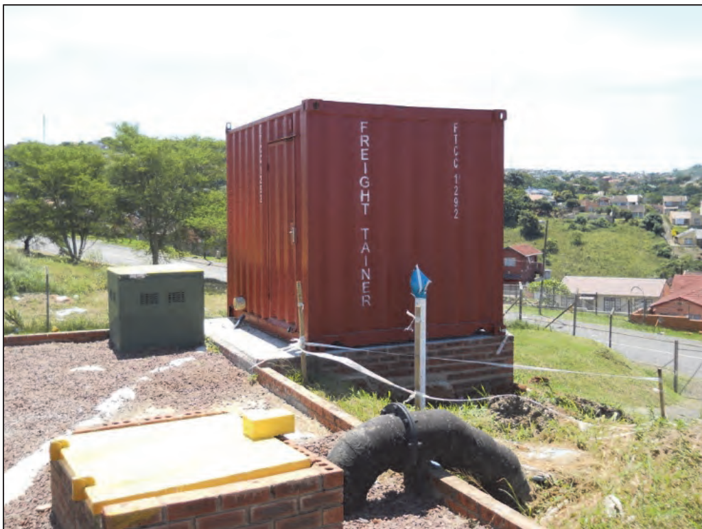
Figure 5-18: Turbine room (steel container) and connection point
