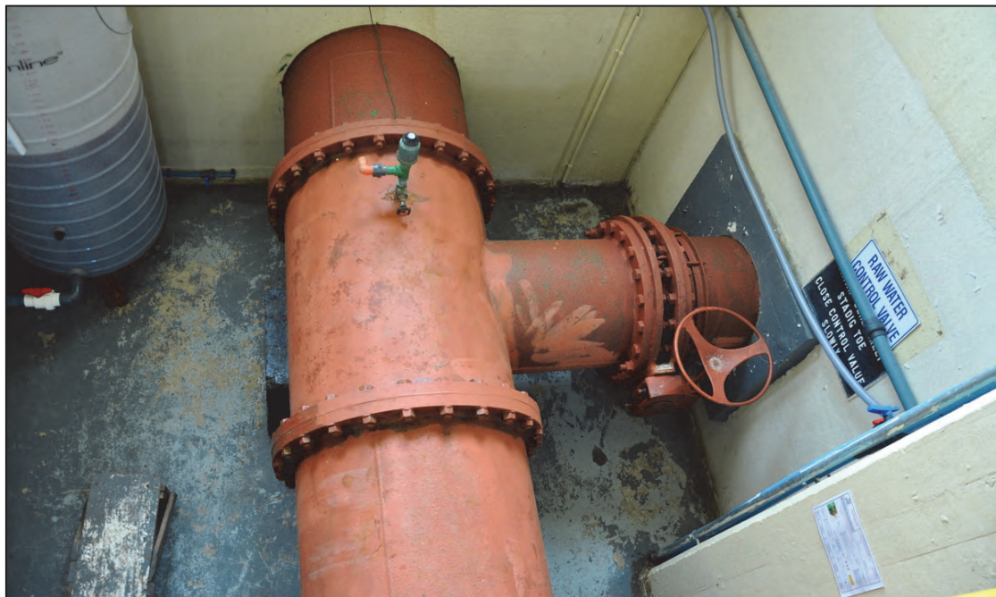
Figure 6-24: Control valve at Nahoon WTW
