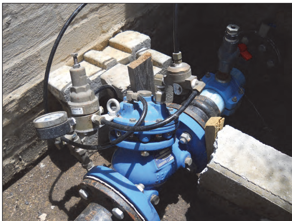
Figure 6-5: Pressure reducing valve (Fraaiuitsig)
