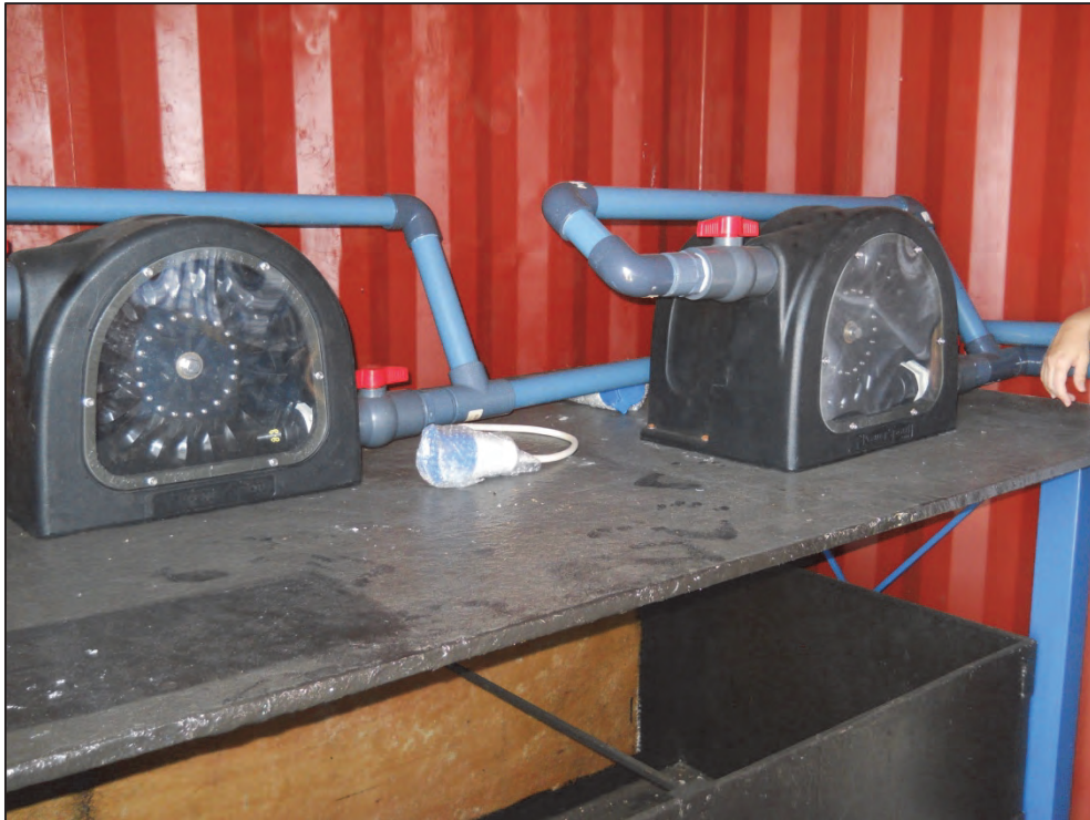
Figure viii: Newlands 2 Reservoir hydropower installation
