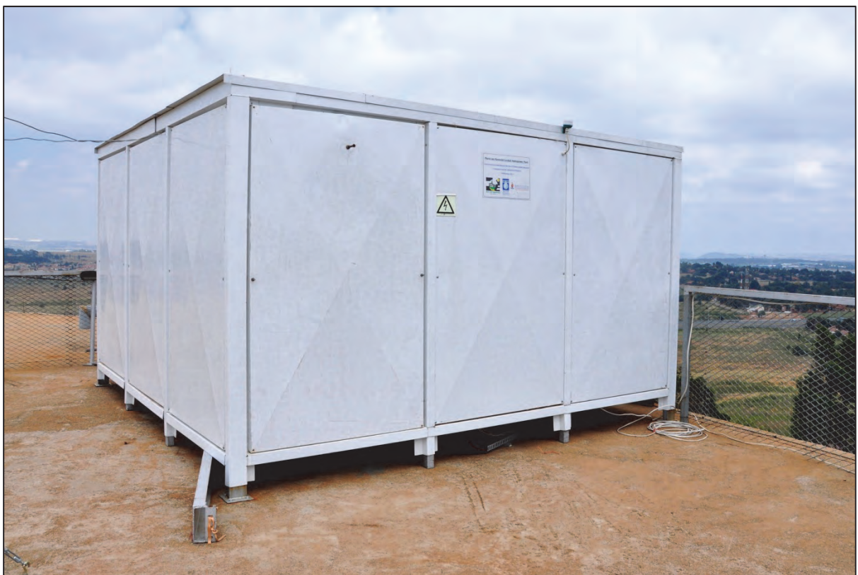
Figure 3-49: Pierre van Ryneveld turbine enclosure
