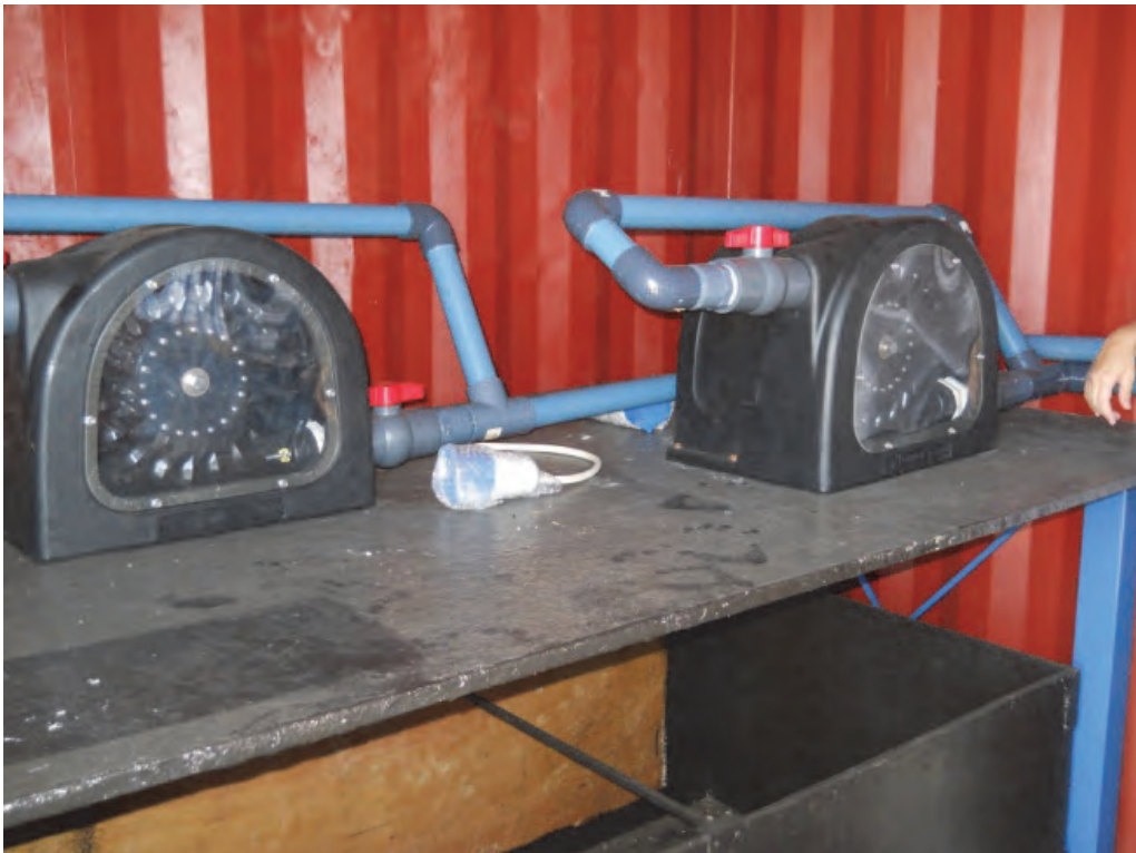
Figure 5-21: Installed turbines in turbine room
