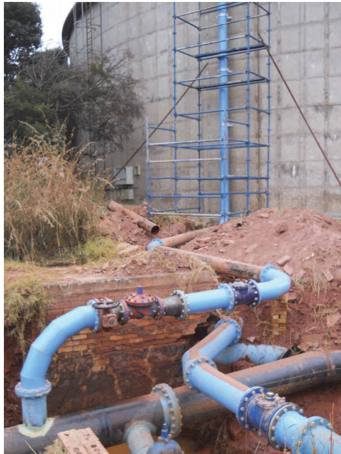
Figure 3-56: Pipework for hydropower installation
