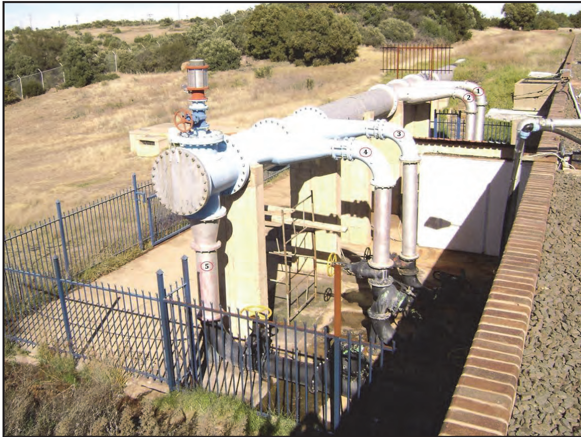
Figure 4-7: Inlet manifold at Brandkop Reservoir (with 5 branches)
