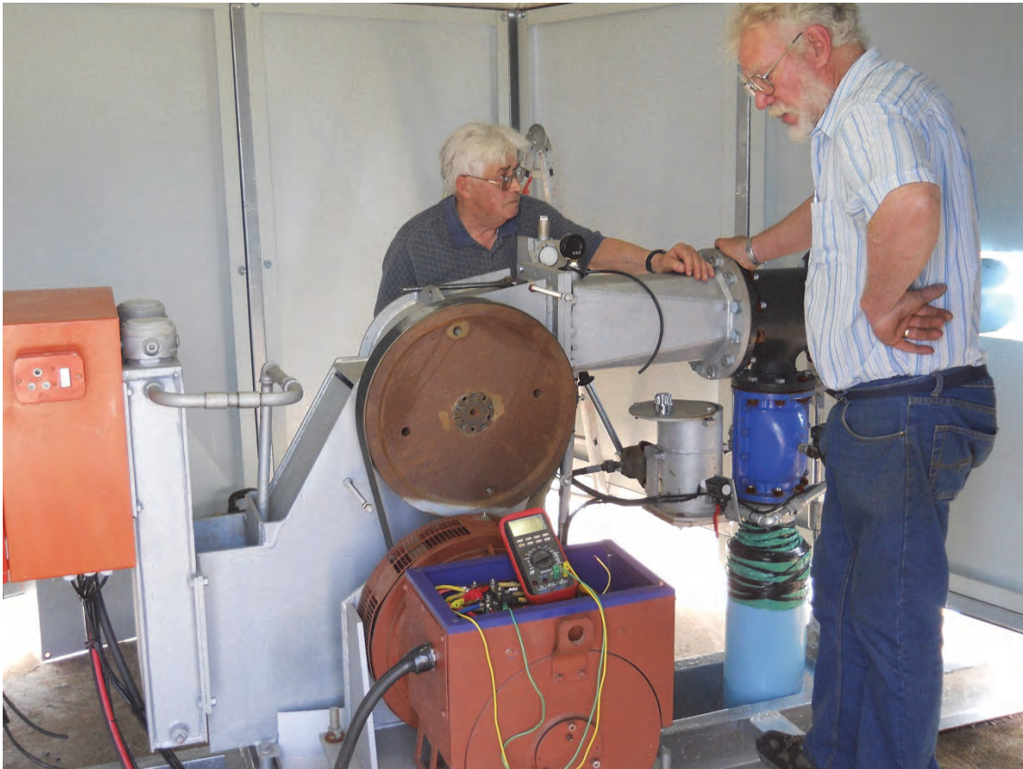
Figure 3-70: Commissioning of hydropower plant
