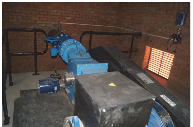
Figure 4-57: Turbine with automatic regulating valve
