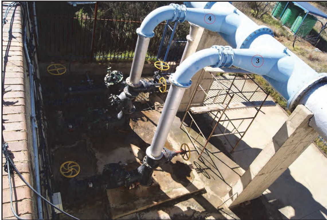
Figure 4-9: Control valves (branches 3, 4 and 5) at Brandkop Reservoir inlet
