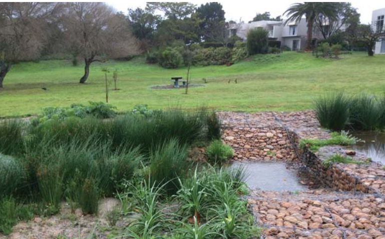
Figure 18. Gabion weirs and indigenous planting effectively address severe channel incision and erosion in this suburban Cape Town stream. (Credit: Liz Day)
