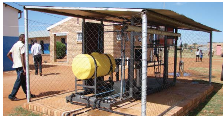
Figure 4. WRC-funded research projects have led to the development of several small desalination plants for rural communities, such as this plant at Madibogo Primary School, in North West, which is used to treat brackish groundwater. (Credit: Lani van Vuuren)
