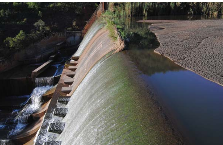
Figure 14. Mapochs Dam, on the Masala River, showing accumulation of sediments. (Credit: Rob Palmer)
