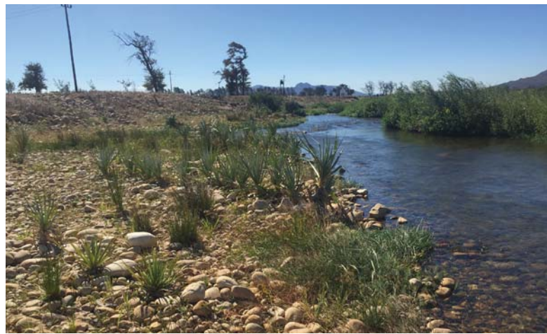
Figure 21. Berg River 'before (top) and after (below)': Rehabilitation of the Berg River following bed and bank erosion as a result of a poorly designed bridge. Rehabilitation is expensive - it is cheaper to avoid degradation in the first place. (Credit: Liz Day)
