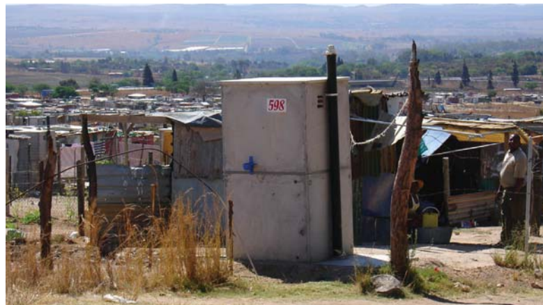
Figure 12. There are an estimated 1.2 million household VIP units in South Africa, located both in rural and urban areas. (Credit top: Lani van Vuuren and bottom: Kathy Eales)
